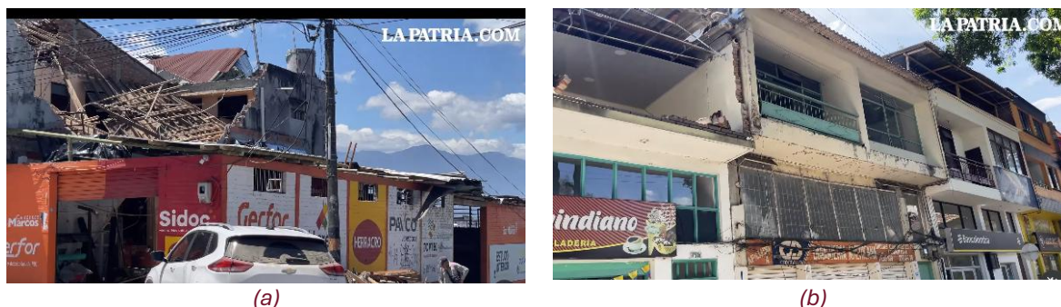
Figure 26 Montenegro, Quindío: (a) damage to roof (b) and facade 21
