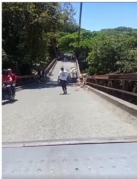
Figure 44 La Unión–La Victoria road corridor is closed due to a bridge collapse 54
