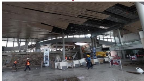
(d) Matecaña International Airport Terminal – detachment of the suspended ceiling and acoustic panel 25
