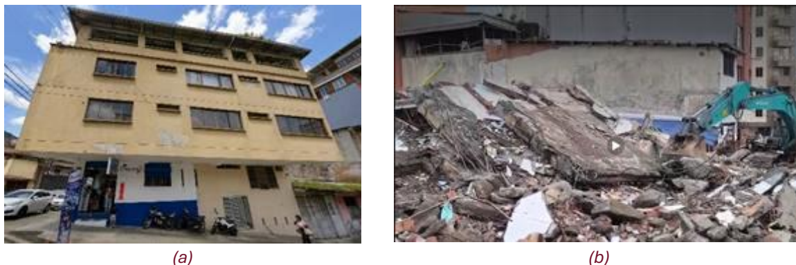
Figure 24 Edificio Naranjito in Buenaventura: (a) building condition before the earthquake; (b) complete collapse following the earthquake 19
