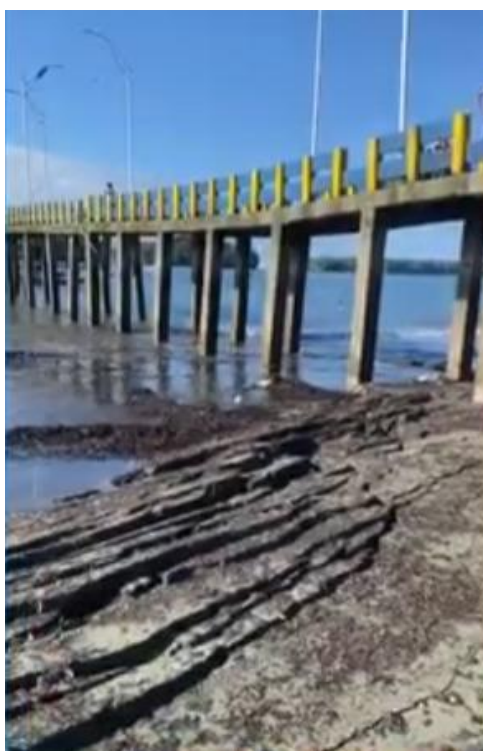
Figure 32 Lateral spreading damage to the Muelle de Juanchaco wharf, Buenaventura, following the 10 August 2026 earthquake 31
