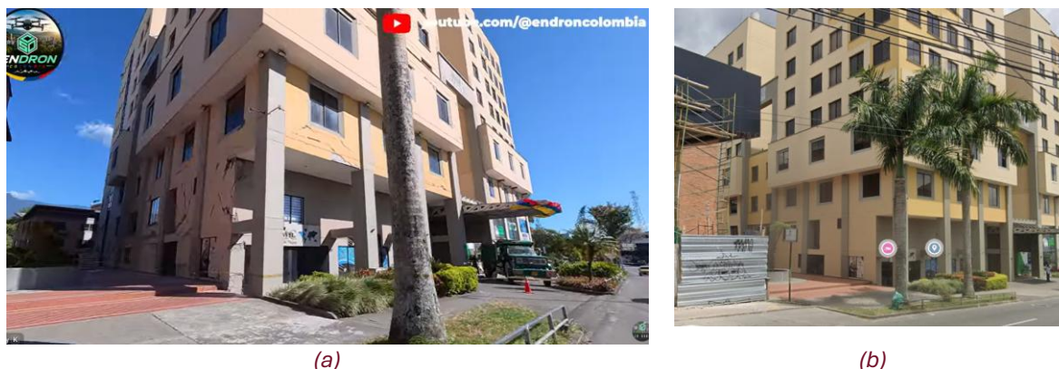
Figure 25 Edificio Armenia Hotel in Armenia: (a) building condition before the earthquake; (b) damage to walls following the earthquake 20
