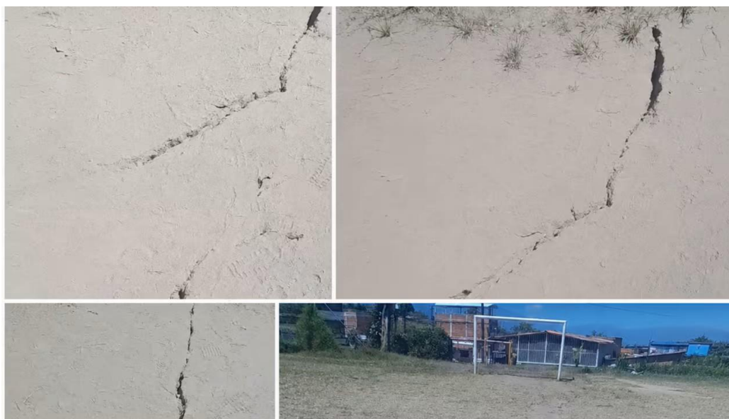
Figure 34 Ground cracking across a levelled football field in the Los Almendros sector, Armenia (Quindío), following the 10 August 2026 earthquake 34
