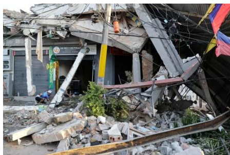
(a) Commercial Corner Block: collapse of a 3-story concrete frame with hollow clay block infill. 23
