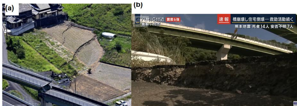
Figure 17. (a) Vertical displacement in the Kyushu Expressway overpass in the foreground with cracks in the adjoining farm in the background 25 , and (b) vertical displacement of the ground observed in the field (and looking up at the overpass) 26
