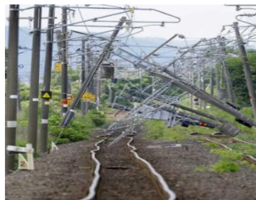
(b) Collapse of utility pole and deformation of railway Between Ogawa and Arisa stations on JR Kagoshima Line ( Link 104 )
