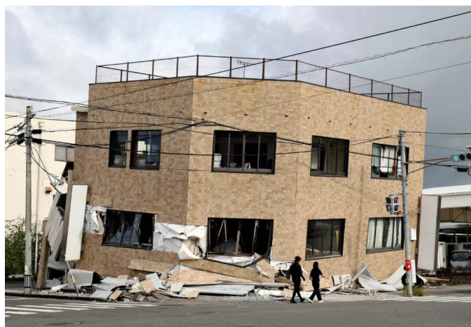
Figure 40. soft storey damage of two-storey building
