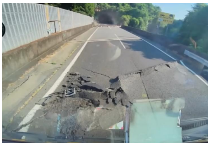
Figure 51. Road damage ( Link 100 )
