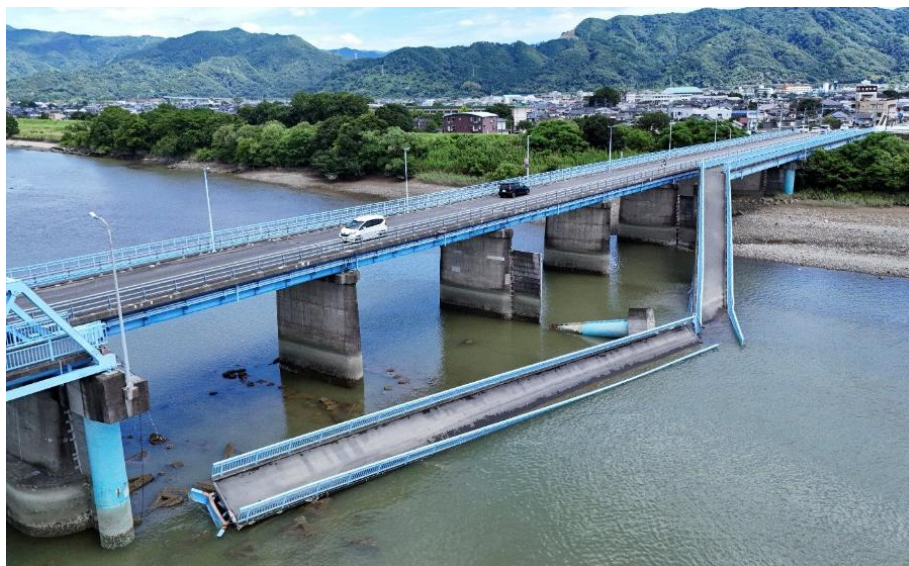
Figure 50. An aerial drone view shows a damaged bridge in Yatsushiro after a magnitude 7.1 earthquake struck Kumamoto Prefecture in southern Japan ( Link 98 )
