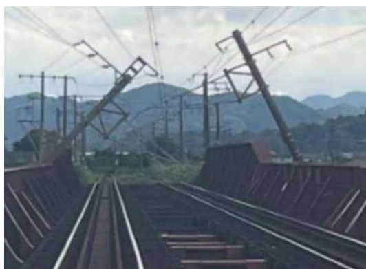
(a) Utility pole damage observed between Ogawa and Arisa ( Link 103 )
