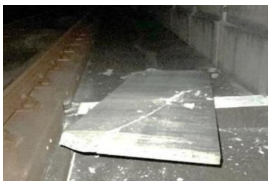
Figure 55. Noise barrier collapse between Kumamoto and Shin-Yatsushiro ( Link 105 )
