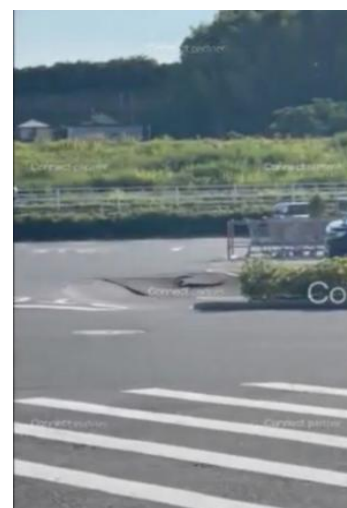
b) Carpark damage ( Link 46 )
