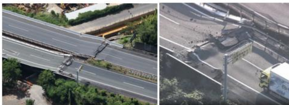
Figure 48. Damage to Kawada Brid ( Link 95 )
