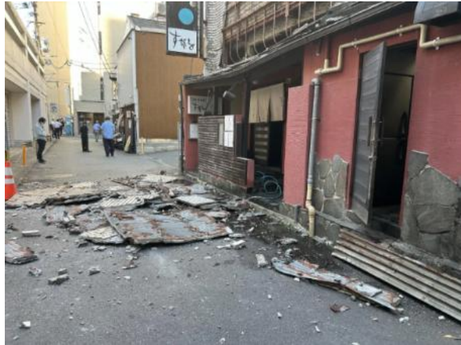
Figure 30. Facade linings losing bonding to exterior walls in a commercial area ( Link 47 )
