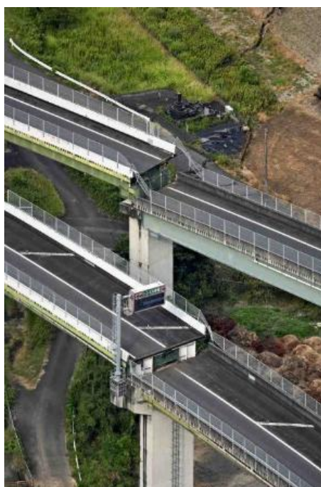
Figure 47. About 1.5 m drop in a bridge deck ( Link 93 )
