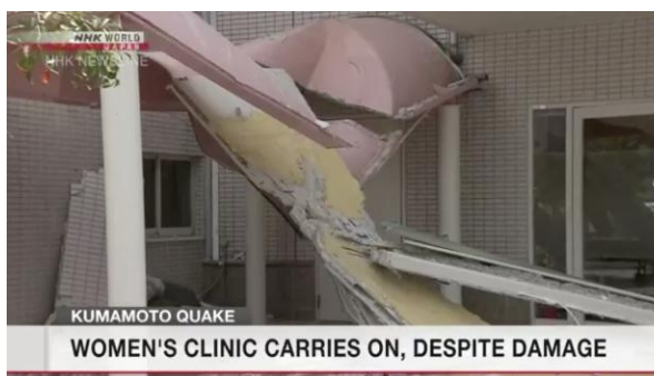
(a) Exterior canopies damage
