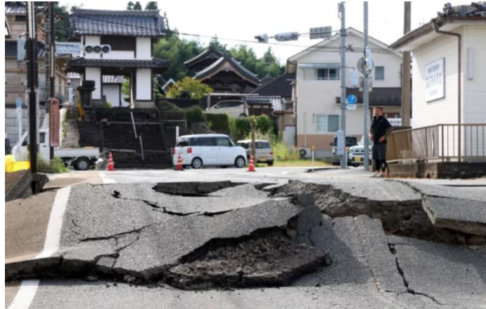
Figure 52. road collapse in Ogawa Town ( Link 101 )
