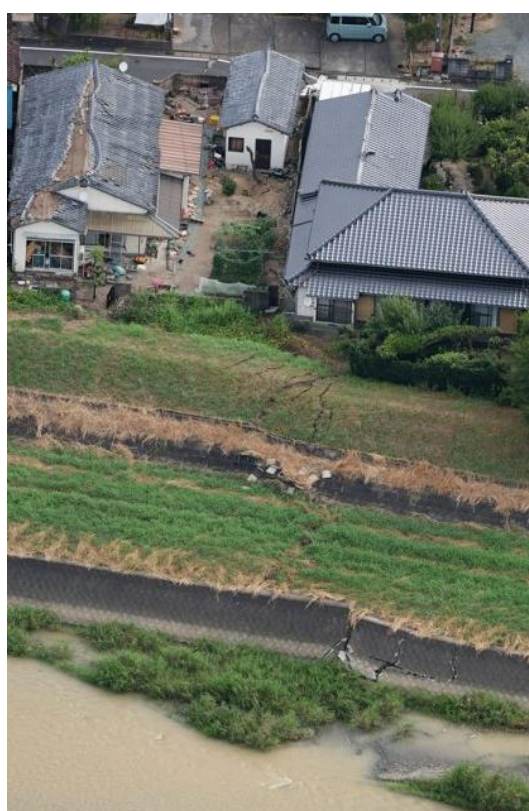
Figure 26. Surface expression of the suspected active fault associated with the 2026 Kumamoto Earthquake sequence, showing visible ground rupture and displacement causing levee cracking in Hikawa, Yatsushiro District (Source: Asahi Shimbun 38 )
