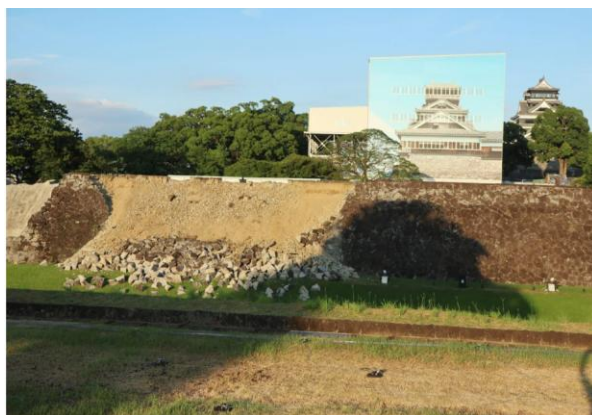
Figure 32. Partially collapsed stone walls at Kumamoto castle.
