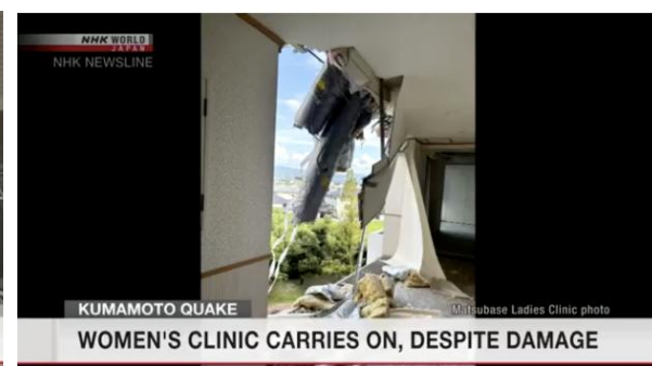
(b) Wall damage
