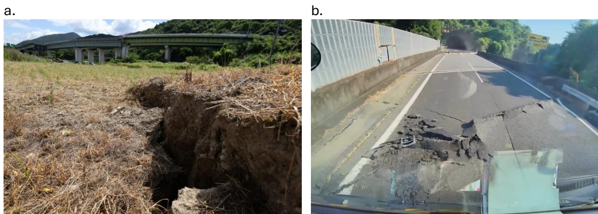
Figure 19. a) A close up of the rupture in Figure 17 and 18 28 b) A crack by the Ohirayama Tunnel entrance, 150 m from the site at Figure 19a
