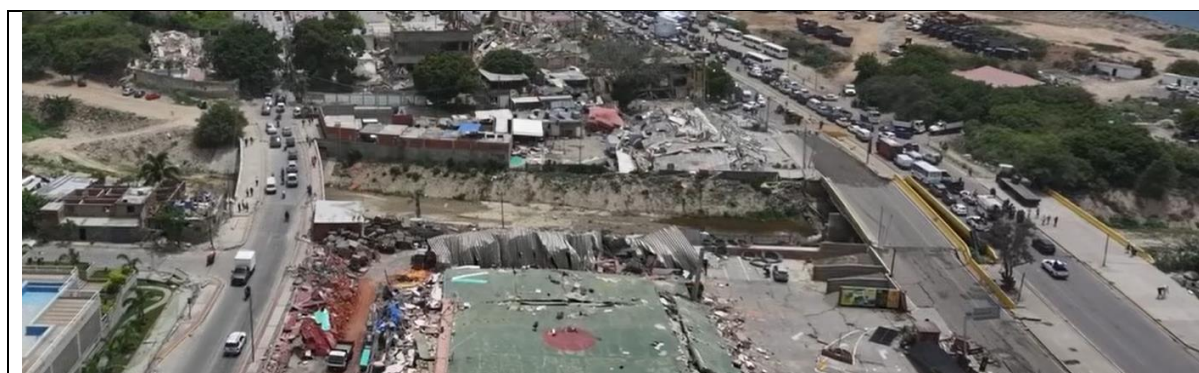
Figure 47. Settlement of approach soils at bridge crossing Rio San Julian (10.619N,-66.851E).
