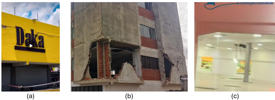
Figure 38. Further damage to commercial buildings in San Felipe: (a) horizontal crack along the display wall; (b) infill wall damage; (c) exposed ceiling system failure.
