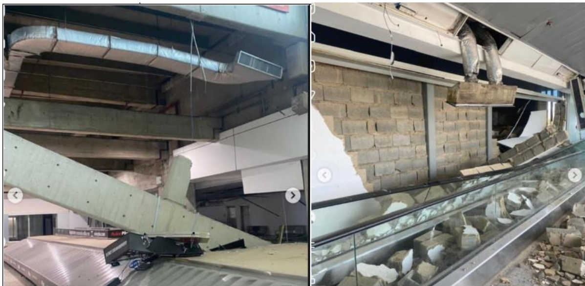
Figure 51. Loss of support of precast beam (left) and infill wall and building services collapse (right) at Simón Bolívar International Airport ( Social Media )
