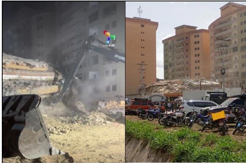
Figure 24. Images of the collapsed tower four at the Bosque Lindo in Turmero, Aragua ( terremotovenezuela , Social Media , Media ).
