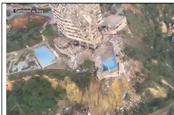
Figure 48 (left). Failure of fills supporting at North corner of a building at Catia La Mar (10.611 N, - 67.008E).
