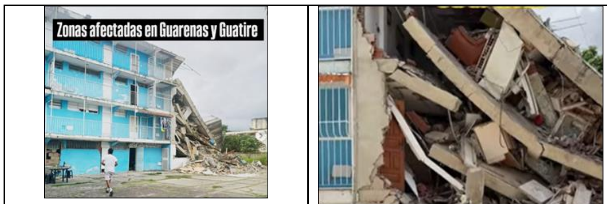
Figure 34. Bloque 8 Oropeza Castillo - a 4-storey residential RC and clay masonry building. From photographs and videos, this building is likely either to have been extended or built in more than one stage. Also, there was a water tank at the roof level.
