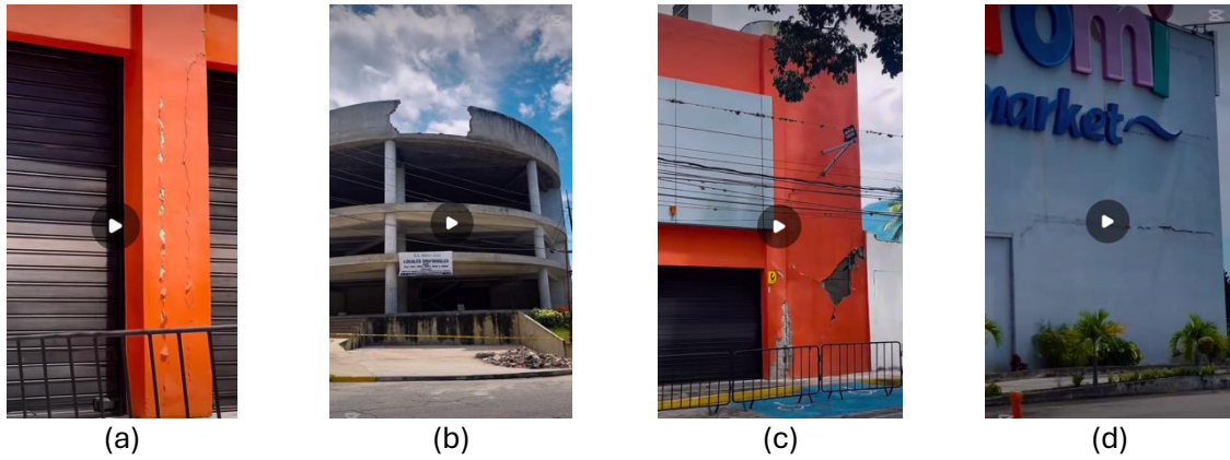
Figure 37. Damage of RC low-rise commercial buildings in San Felipe: (a) concrete cover cracking; (b) cracking in curved wall components; (c) damage of infill wall; (d) separation between infill walls and structural frames.
