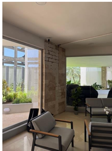
Figure 43. Minor damage to concealed ceiling system in low-rise RC frame buildings at Residencias Atlántica, Tucacas.
