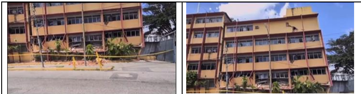
Figure 32. Hospital Risquez showing a ground floor soft-storey.
