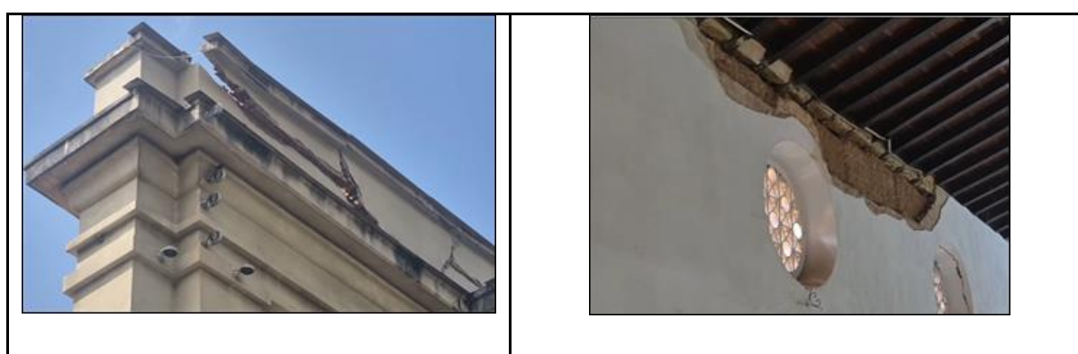
Figure 35. Catedral de Nuestra Señora de Copacabana. This building was built in 1800, using adobe as construction material, with a renovation in 1950. It appears to have experienced minor damage, mainly through parapet cracking.
