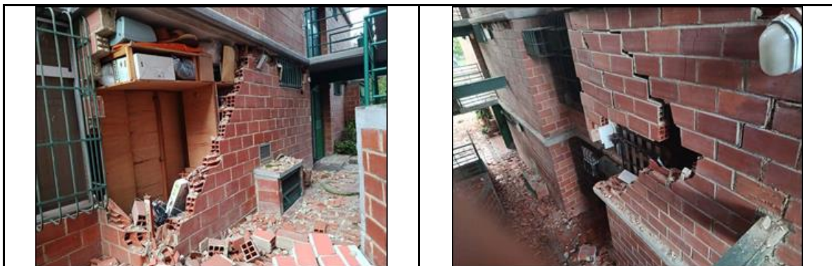
Figure 33. Residencias El Tablon – showing an unreinforced-unconfined clay masonry wall in the 4-storey building and shear failures, mainly at ground and first floor levels.
