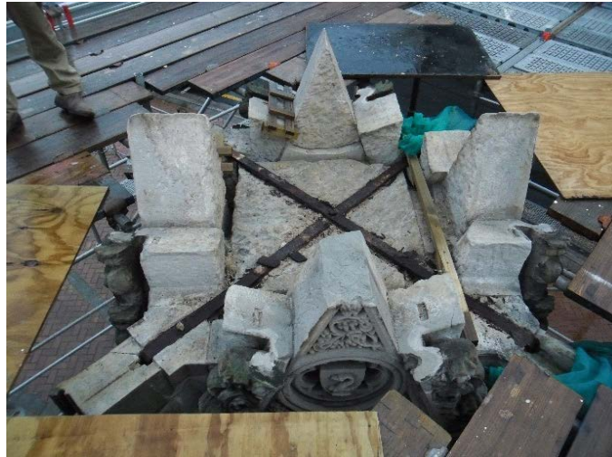
Figure 7. Dismantling revealing original corroded tie bars.
