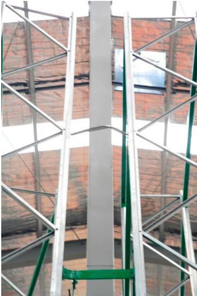
Figure 7 Evidence of impact damage to a racking system from the adjacent building structure
