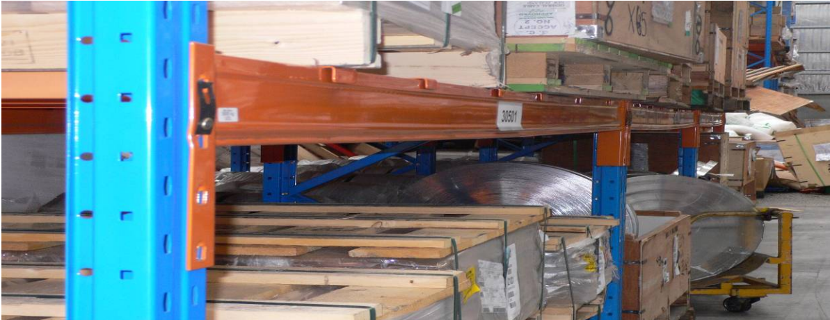
Figure 3 Beams deflecting under approximately half of the specified maximum UDL
