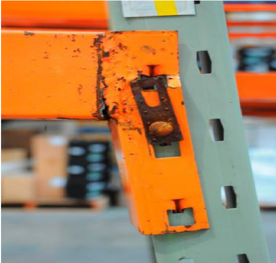
Figure 5 Failure of welded joint between beam and bracket
