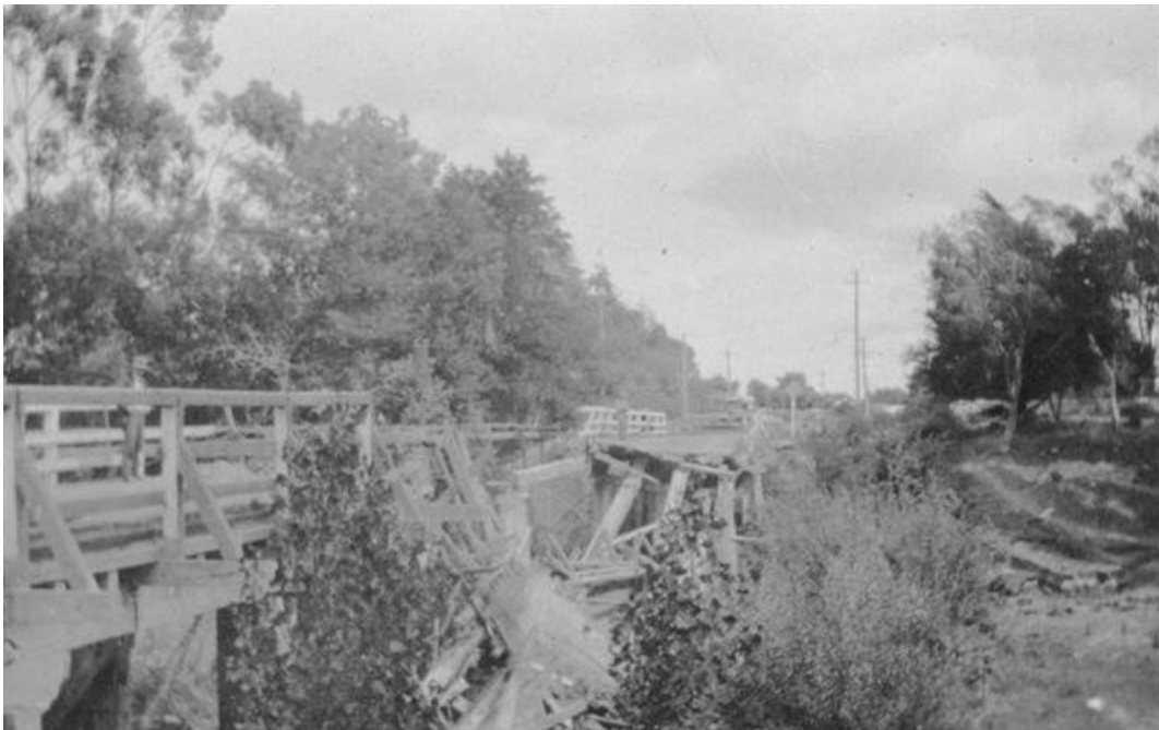
Figure 10. The Havelock North Bridge was one of many bridges in the region damaged during the earthquake.
