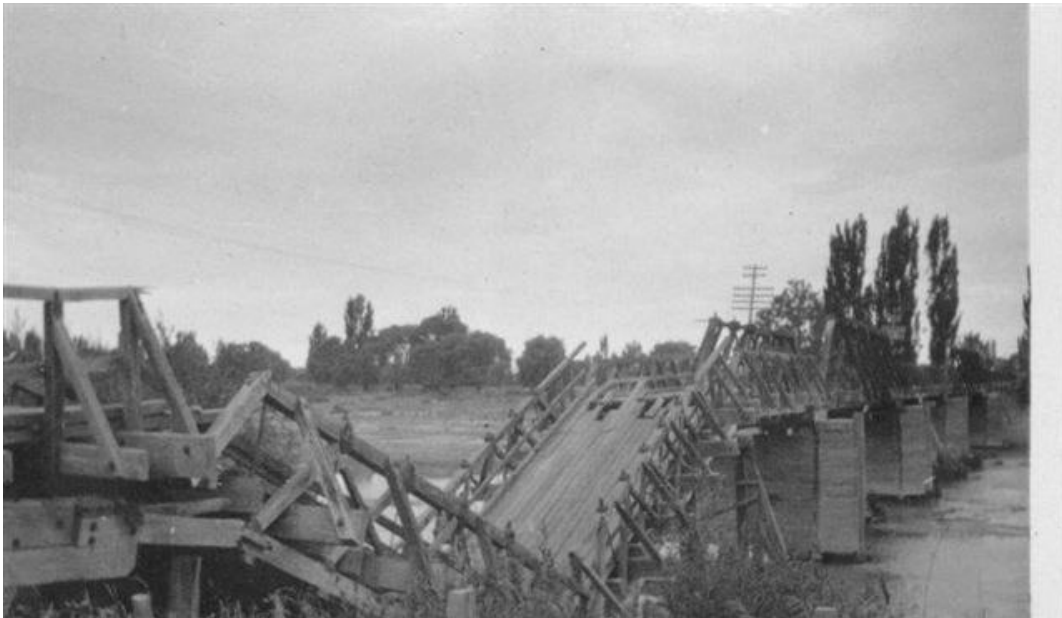
Figure 8. Because of its strategic importance to the Redclyffe Substation, damage to the Redclyffe bridge at Waiohiki near Taradale added to the disruption of power supply services.
