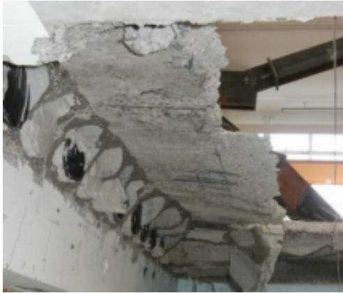
(e) The remaining topping and ends of the hollowcore units after collapse.
