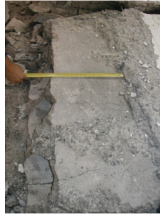
(f) The delaminated topping on the failed unit.
