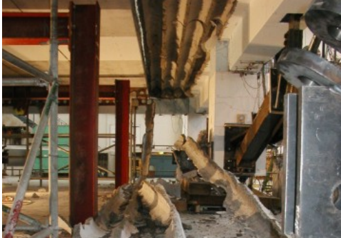
(a) Failure of the first hollowcore unit
