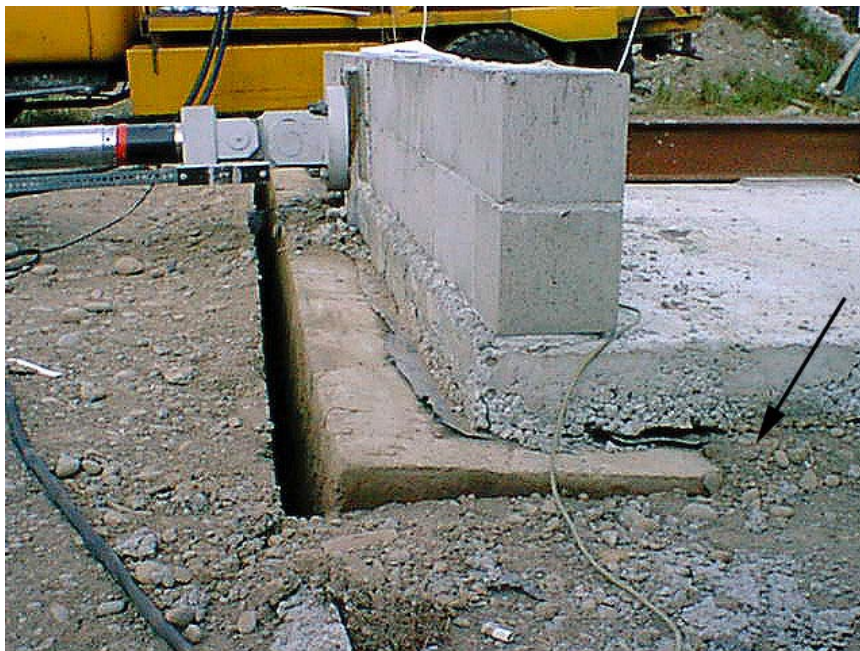
Figure 9. Rotation and uplift of foundation beam for Test 2. Arrow indicates location of the passive soil wedge.
