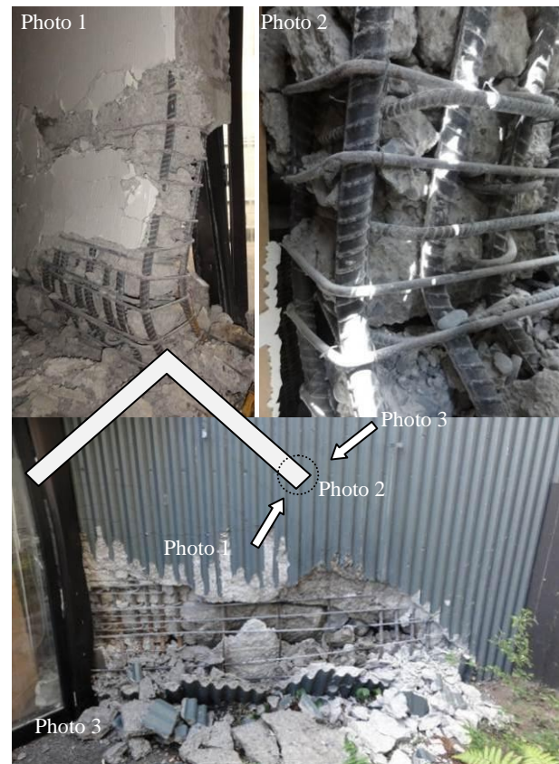
Figure 33: Seven-storey 1980s office block with significant compression failure of the V-shaped RC shear wall.
