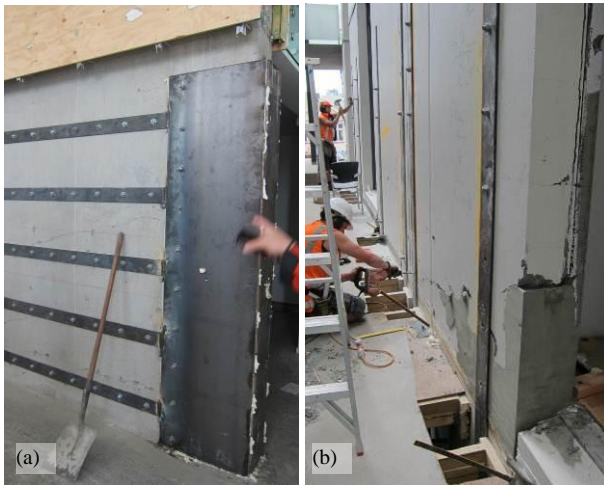
Figure 69: Emergency stabilisation repair of RC walls with a) buckled boundary longitudinal bars with inadequate confinement ties; b) fracture boundary longitudinal bars across a single cracking line.
