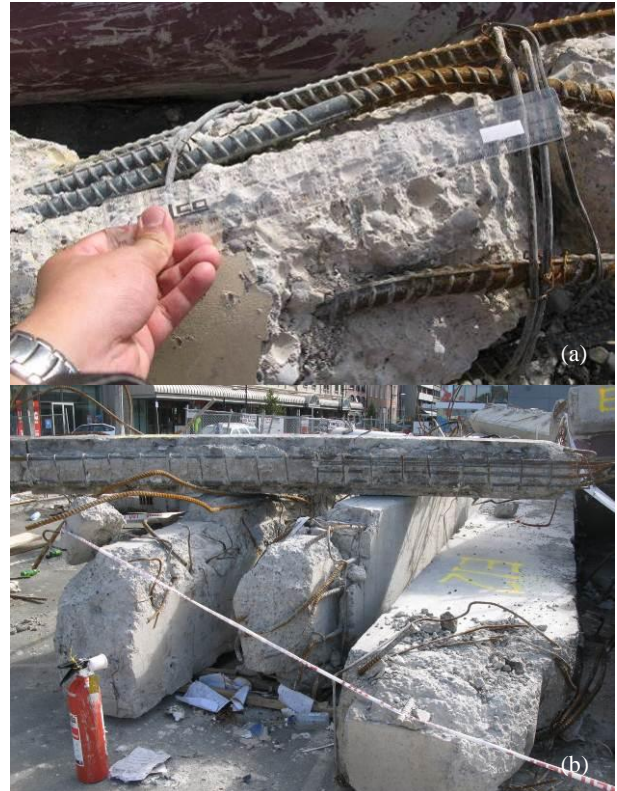
Figure 56: Post-demolition inspection of the RC frame elements: a) RC column with R6 spiral ties at 250 mm centre and six-HD20 longitudinal reinforcement.
