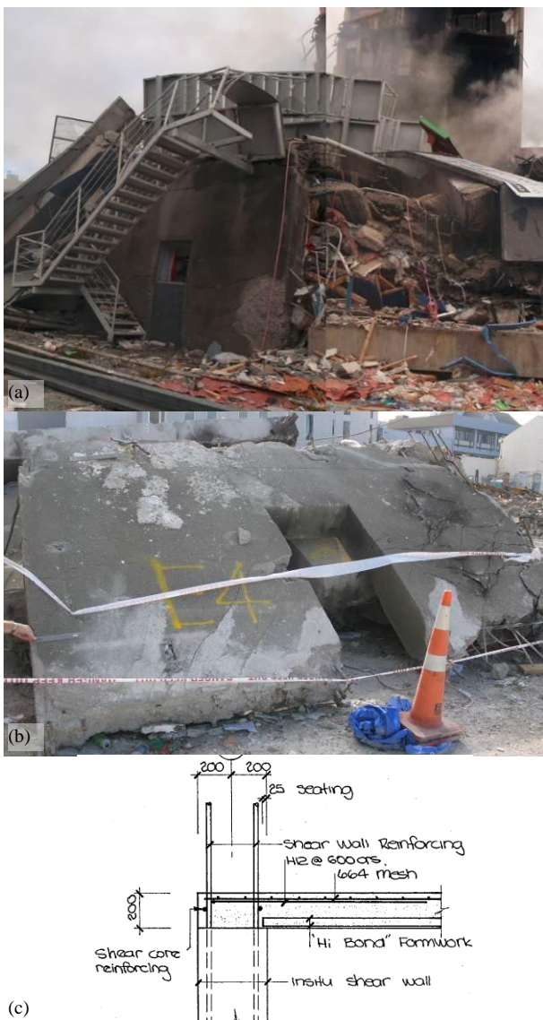
Figure 55: Coupled walls on the Southern side: a) the coupled walls remains intact on the Ground Floor with limited flexural or shear cracking; b) All six pairs of the coupled-walls were accounted for during a post-demolition inspection – limited damage were observed on these walls; c) the connection detail of slab-to-coupled walls.
