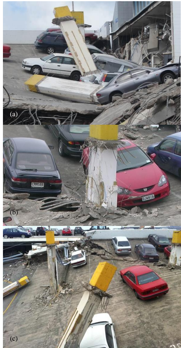
Figure 38: Punching shear failure of a 5-storey post-tensioned flat-slab and columns building. (Photograph (c) is courtesy of David Swanson).
