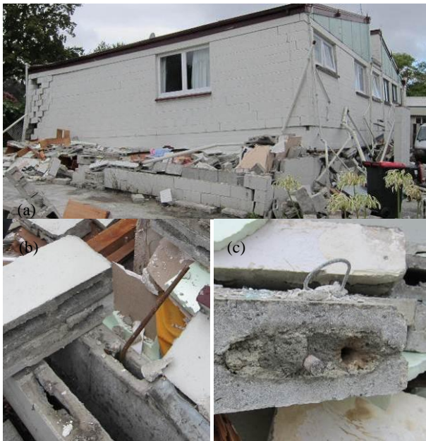
Figure 23: a) Soft-storey collapse of a 2-storey residential RCM building. (b-c) Anchorage pull-out failure of the lapped vertical reinforcement.
