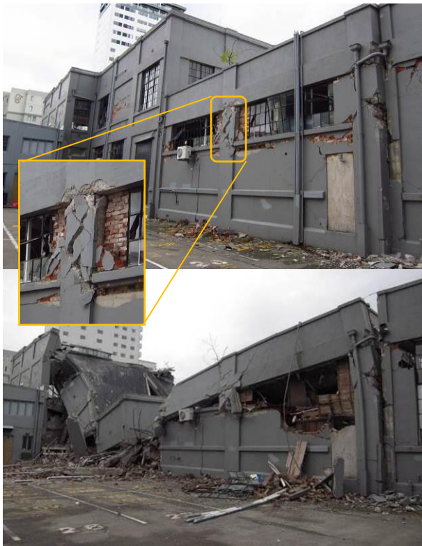
Figure 20: Reinforced concrete frame buildings collapse/damage patterns: Pre-1930s three-storey RC frame with masonry infill a) Survived the 22 February 2011 M_w 6.2 earthquake; b) Collapsed after the 13th June M_w 6.0 aftershock; insert: short column failure.
