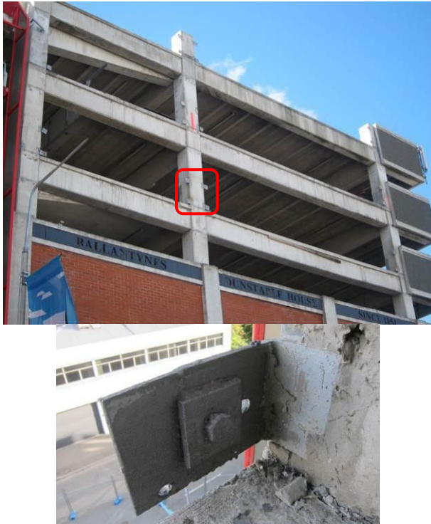
Figure 42: Failed precast concrete façade panels “welded and slotted-bolt” connection (construction error).
