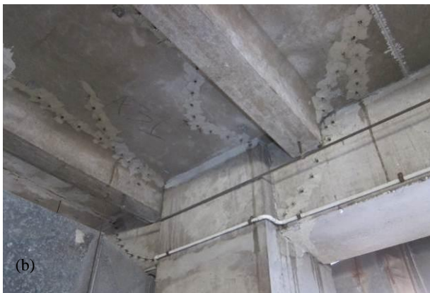
Figure 29: Ductile RC perimeter frames building with beams hinging, floor slab damage and collapsed precast staircase at upper levels (8 th to 11 th floor). Photo (b) is showing the crack repair done after the 4 September earthquake.
