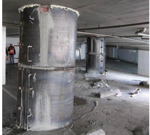
Figure 67: Emergency stabilisation repair of the columns with axial-shear failure. See Figure 60 for the pre-repair condition of the columns.
