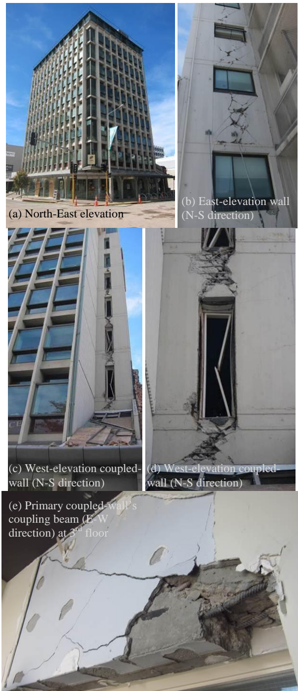
Figure 19: a) Seven-storey 1960s coupled-RC walls building with significant damage on the coupling beams. b) Shear walls damaged at East elevation; c-d) Coupled-wall damage at the West elevation; e) Damaged coupling beam at the internal coupled-walls (East-West direction).
