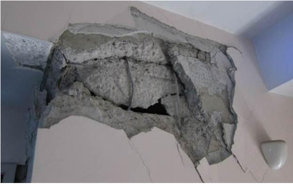
Figure 18: Compression zone failure of pre-1970s RC walls. Photo is taken from the ground floor wall of an early 1960s 9-storey RC building.
