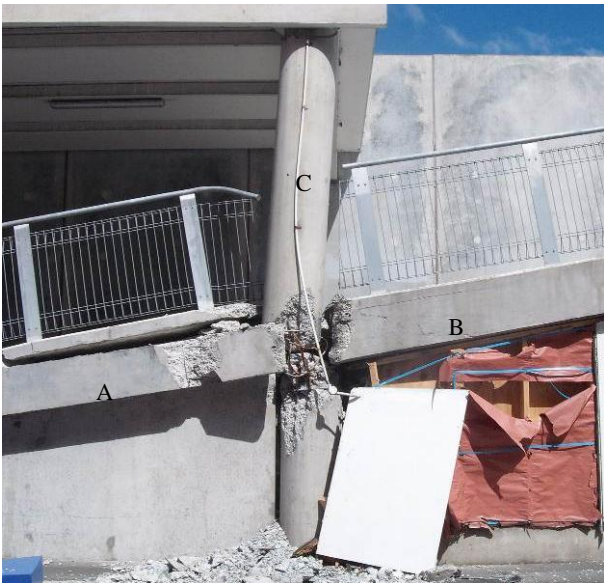
Figure 39: Lack of displacement allowance for ‘simply-supported’ elements such as car park ramp leading to a column shear failure.
