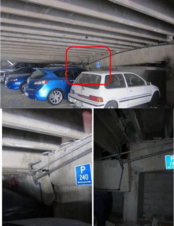
Figure 37: Localised collapse and loss of gravity support at the 1st floor at the 5-storey car park due to corbel failure.
