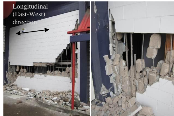
Figure 21: Flexural-shear damage of a RC masonry infill wall within two-storey RC frames.
