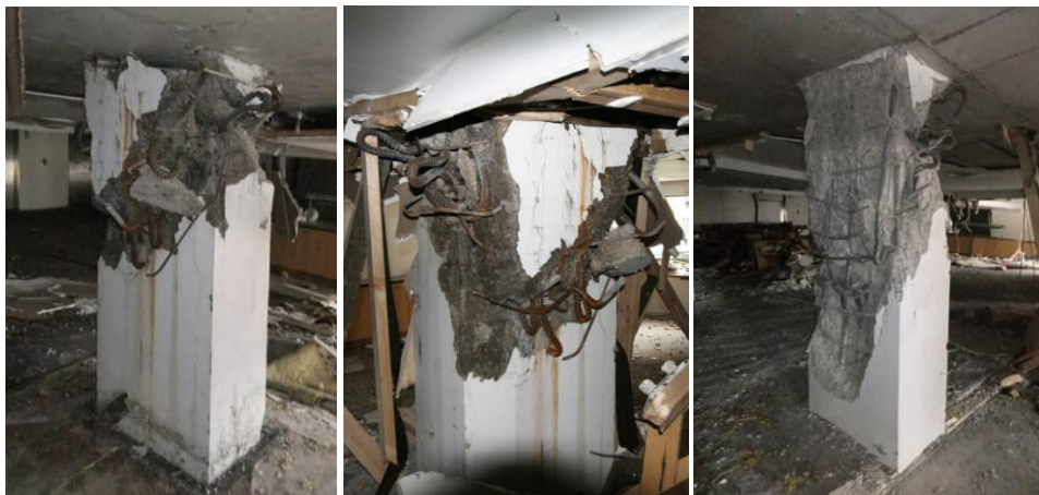
Figure 60: Grand Chancellor Hotel: The shear-axial failure of the RC columns below the transfer girders at Level 10 and 11.
