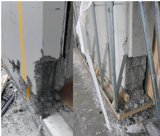
Figure 34: Bar buckled and fractured in lightly reinforced slender RC shear wall: a) North-South Wall; b) East-West Wall.
