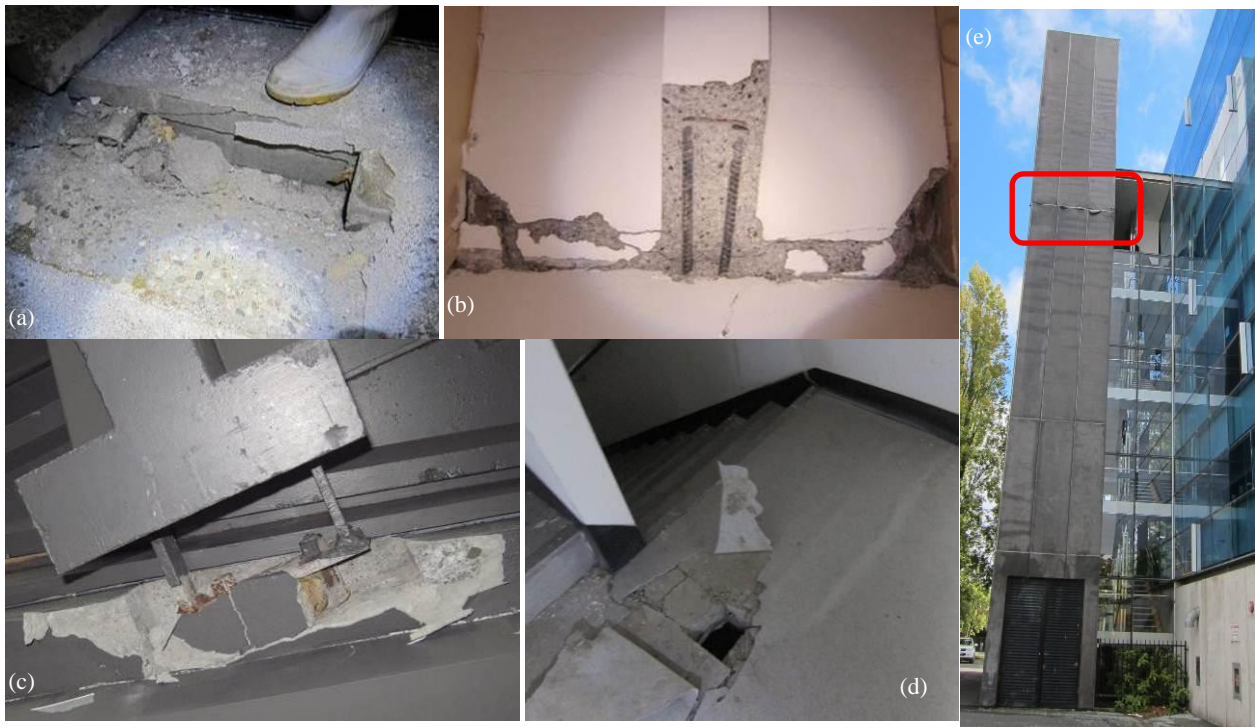
Figure 62: Typical ‘severe’ top and bottom landing damage of precast concrete staircase in multi-storey buildings.
