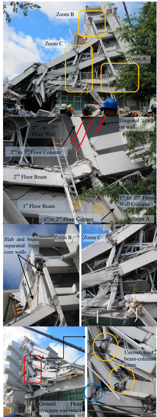
Figure 50: Various failure mechanisms observed on the Northern elevation of the collapsed PGC building.
