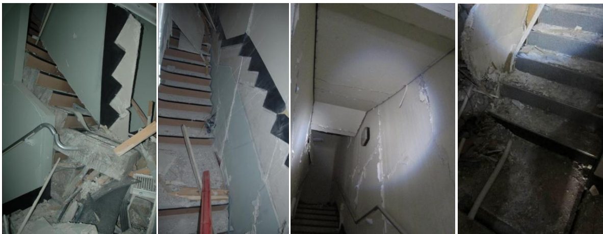
Figure 64: Collapse of one out of two internal scissor staircases in a multi-storey RC frame building. The staircase was under repair work for the damage sustained in the 4 September 2010 earthquake.
