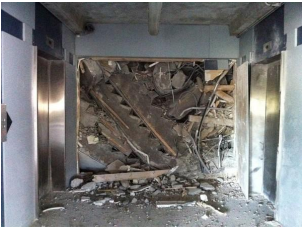
Figure 61: Collapse of precast concrete staircase in multi-storey buildings.
