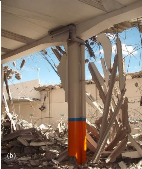
Figure 40: Lack of displacement allowance for ‘simply-supported’ elements leading to failure and collapse of car-park ramp: a) Unseating of hollow core unit at one-simply supported end; b) Collapse of one bay of ramp, possibly due to compressive buckling and pounding with the abutment. Photographs are courtesy of John Marshall [38].
