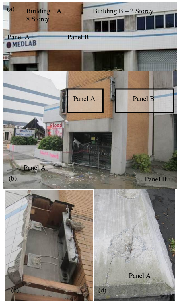
Figure 41: Failure of heavy precast concrete panel connections: a) Panels prior to the earthquake; b) collapse of the panel at the entrance; c) Close-up view of the two anchorage types; d) Pull-out concrete cone on the panel.
