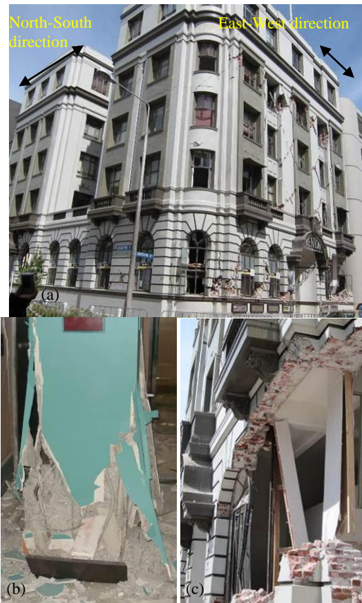
Figure 27: The 6-storey Kenton Chambers (1929) with perimeter URM walls and interior RC frames.
