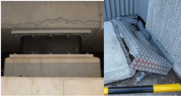
Figure 44: a) A Lead-Rubber-Bearing isolation device with near zero residual deformation (compared to 50mm after the 4 September earthquake); b) The seismic moat cover on the ground level indicates significant lateral movement during the earthquake.
