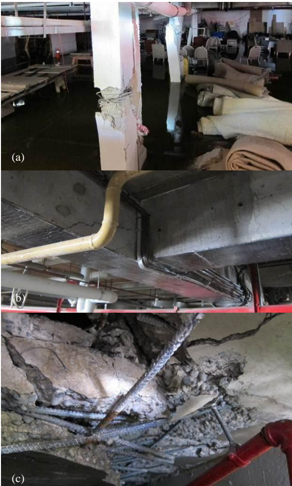
Figure 32: Vertical irregularity resulting in (a) severe basement columns shear-axial failure; (b) transfer beam repair and damage; (c) Ground floor transfer slab failure.
