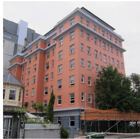
Figure 26: The 8-storey St Elmo Courts (1935) suffered heavy masonry infill walls damage.
