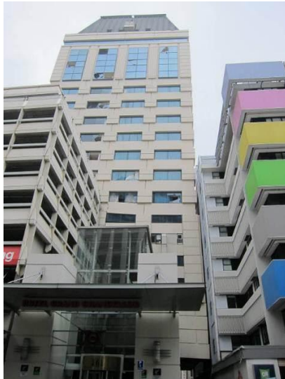
Figure 57: The Southern elevation of the Grand Chancellor Hotel, with a distinct 200 to 400mm lean towards the East (right) side immediately after the 22 February 2011 earthquake.
