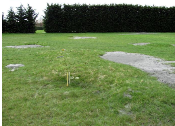
Figure 4: A liquefaction blister, ~300 mm high. The ejected liquefaction sediment to the right of the blister was caused by excessive extension of the topsoil, causing the blister to 'burst'.
