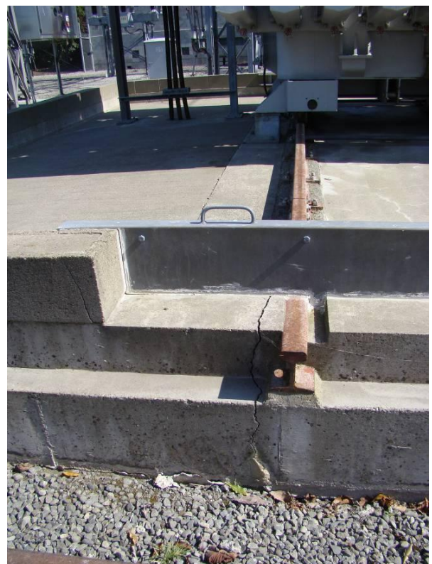
Figure 6: Crack in the bunding (Papanui Substation).
