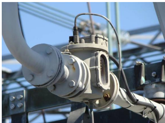
Figure 1: Buchholz relay that is between the transformer tank and conservator.
