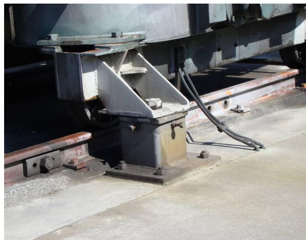
Figure 3: Seismic restraint on transformers (Papanui Substation).
