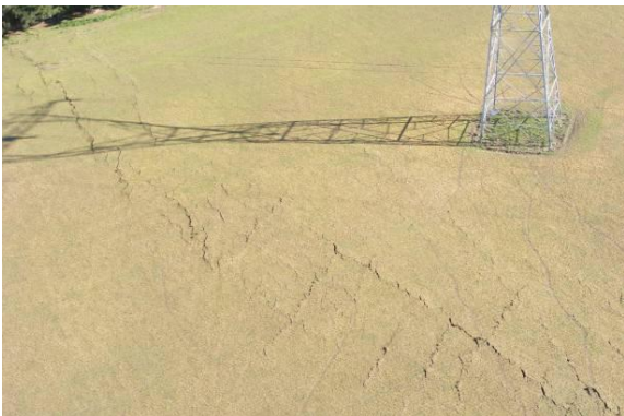
Figure 5: Fault rupture near a 220 kV pylon.
