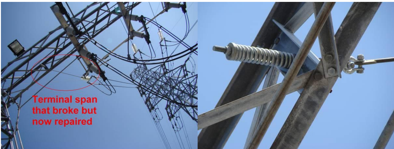
(a) Terminal span showing Phase that failed
