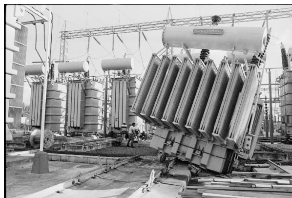
Figure 2: Workmen are dwarfed by a 20-tonne transformer toppled from its mountings at Edgcumbe substation. Photograph taken 4th March 1987 by Evening Post staff photographer John Nicholson (courtesy: Alexander Turnbull Library).
