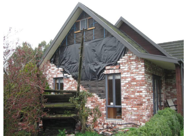
Figure 5: Collapse of recycled brick veneer .
