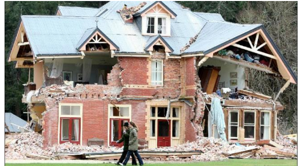
Figure 7: Collapse of double brick veneer house at Homebush (Lyndon Mechielsen, Source: The Australian).
