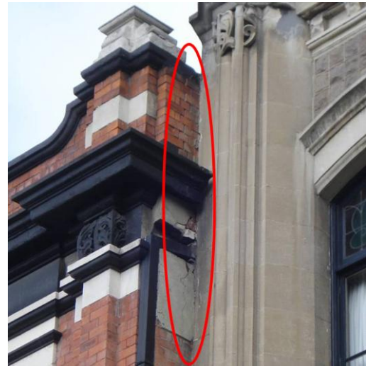
Figure 3: Damage to wall resulting from adjacent facade setback
