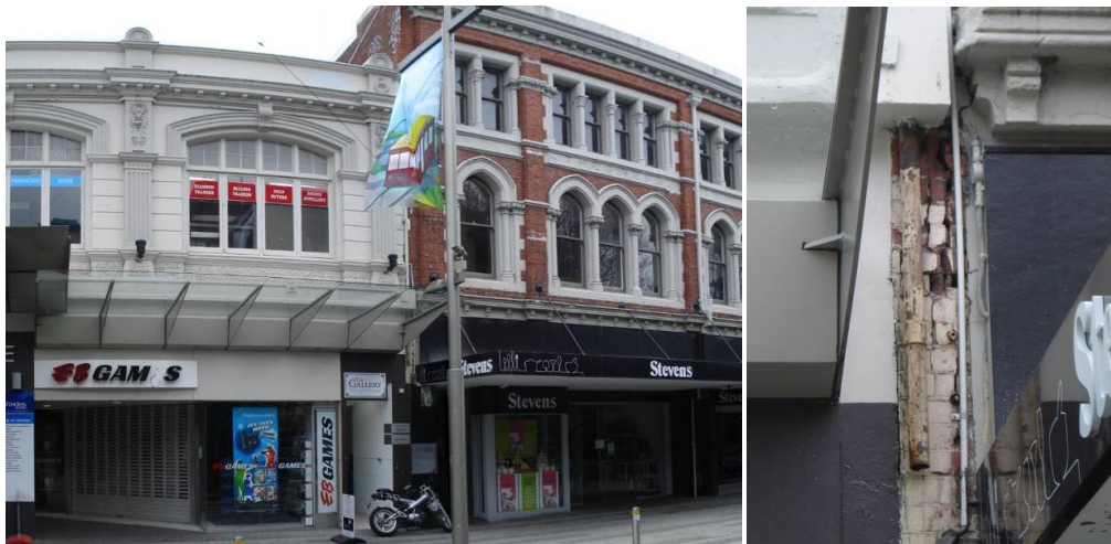
Figure 7: Local crushing of brick between buildings. Left: Building configuration. Right: Magnification of damage between buildings at the first floor.
