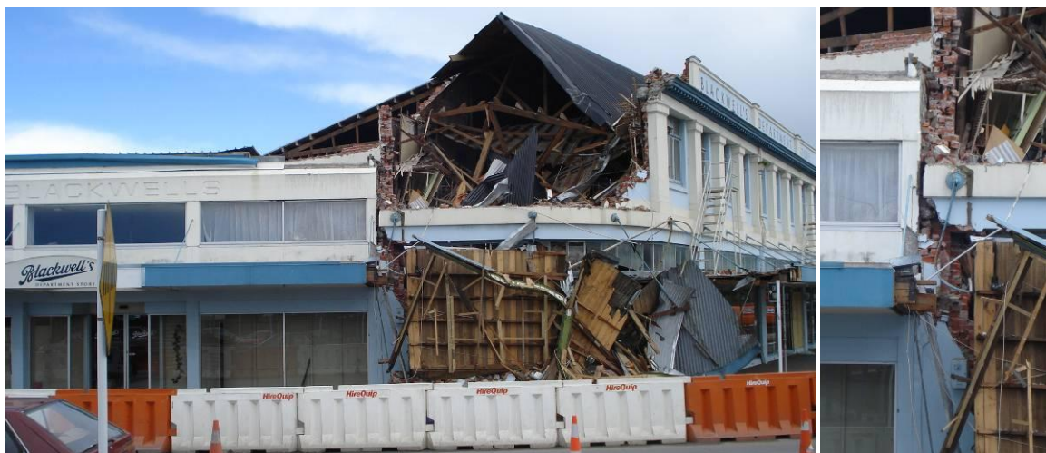
Figure 9: Damaged masonry structure in Kaiapoi. Right: Magnification of damaged building interface.
