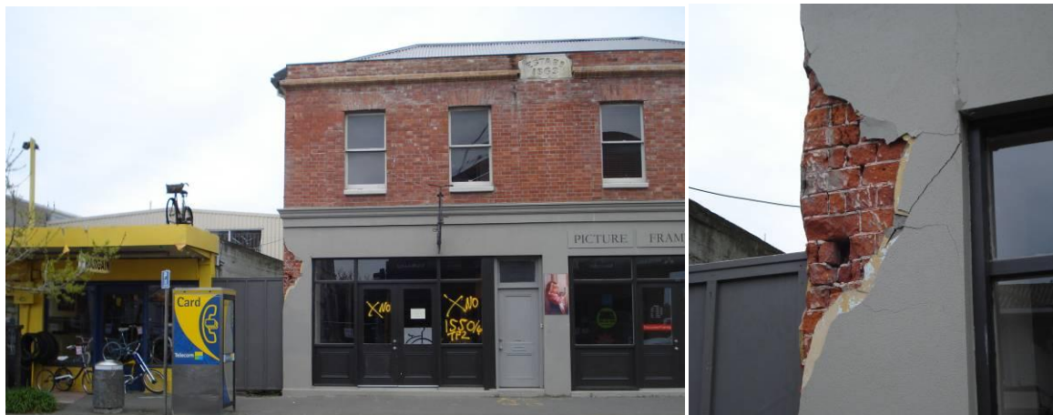
Figure 8: Pounding damage resulting from adjacent fence.
