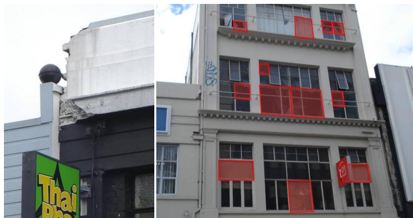
Figure 1: Minor pounding damage. Left: Spalled concrete at building interface. Right: Glazing damage (highlighted) predominately located at the third floor, which coincides with the roof of the adjacent buildings. Cracks are also present at the top of the left hand building.
