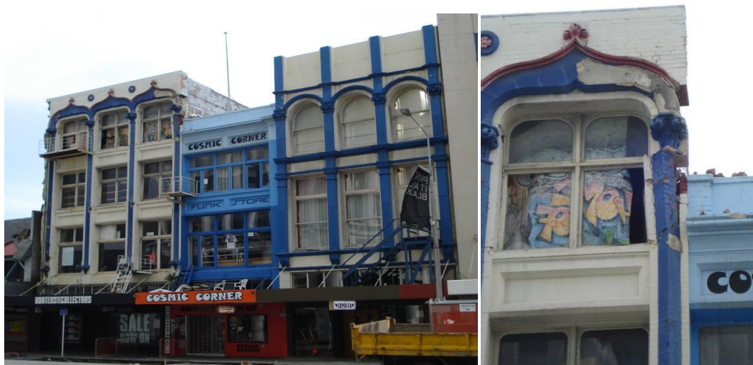
Figure 6: Top floor pounding. Pounding damage has been amplified by the relatively strong window lintel, localising the damage to the masonry below the lintel. Minor damage is present in the adjacent building's parapet. Left: Building configuration. Right: Magnification of damage.
