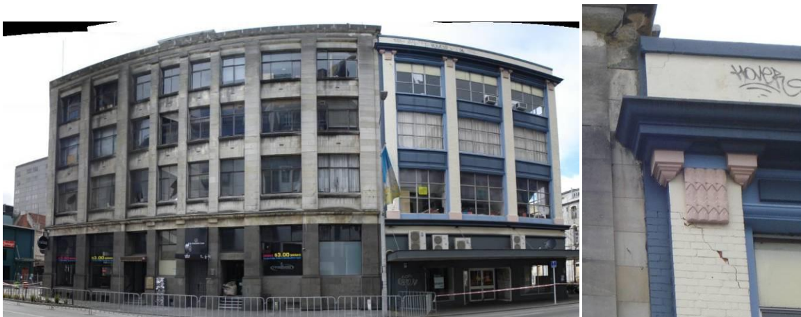
Figure 4: Pounding damage between two four storey structures Left: perspective image of building configuration. Right: Magnification of damage to top of right structure.
