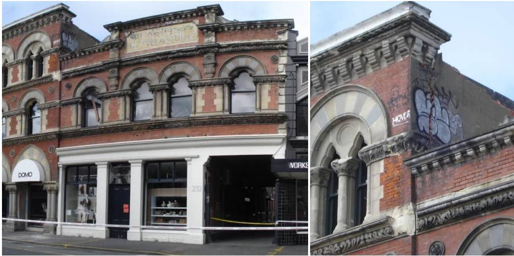
Figure 2: Loss of decorative cladding, and damage to masonry wall partly due to pounding. Right: Magnification of damage at the left building interface.
