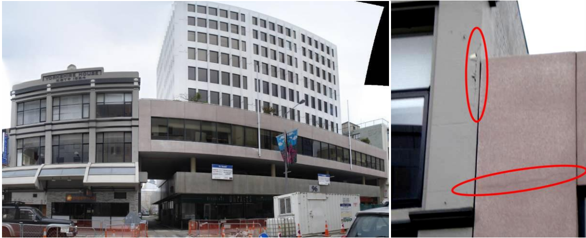
Figure 5: Minor damage resulting from pounding buildings of greatly differing heights. Left: perspective image of building configuration. Right: Magnification of damage at the building interface.
