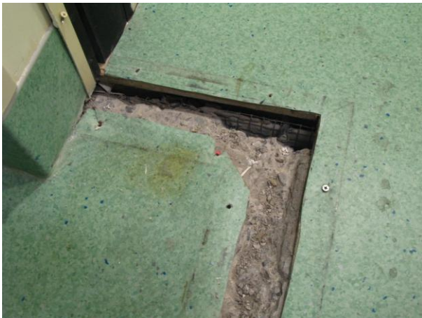
Figure 4: Damage at the seismic gap between the Christchurch Women's Hospital and the Parkside West Building at Level 5 (photo W.Y. Kam)
