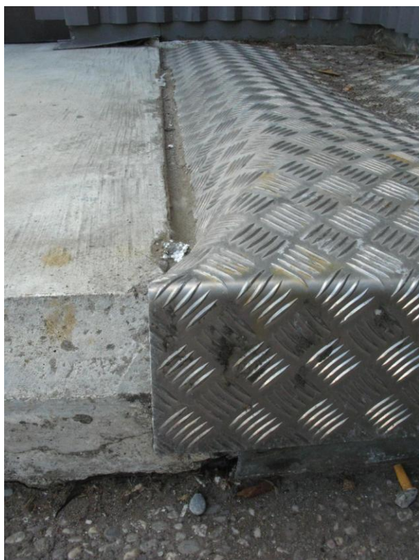
Figure 5: The seismic moat cover plate on ground level at the South corner of the Christchurch Women's Hospital was secured along both edges. (photo W.Y. Kam).
