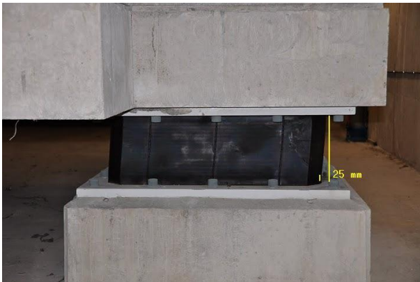
Figure 3: Residual Displacement of LRB at column F-3. (photo F.M. Turner)
