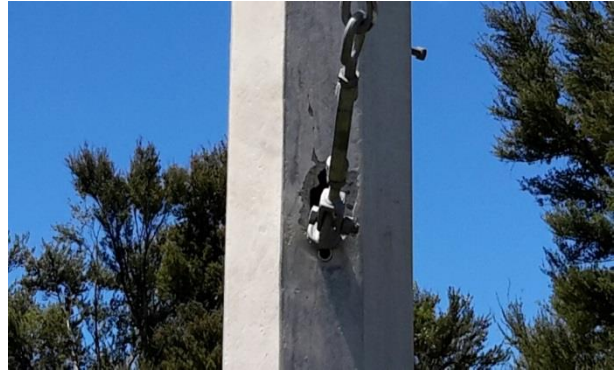
Figure 9: Cracked 66 kV pole.
