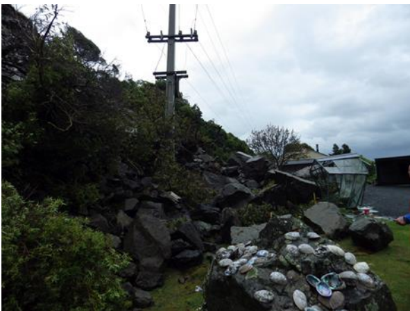
Figure 8: Oaro 33kV pole damage.
