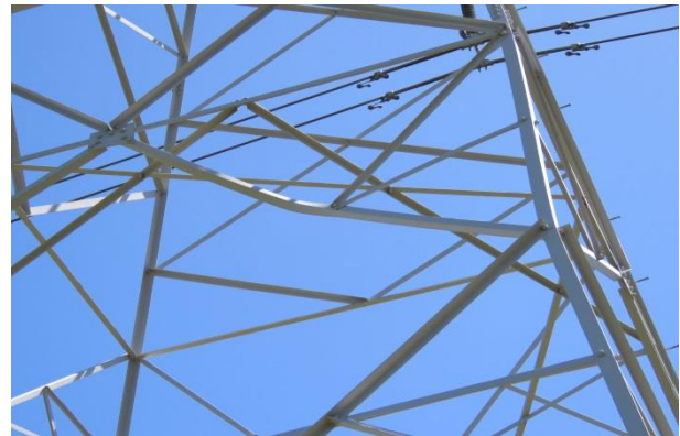
Figure 6: Damaged face of the HVDC Tower.
