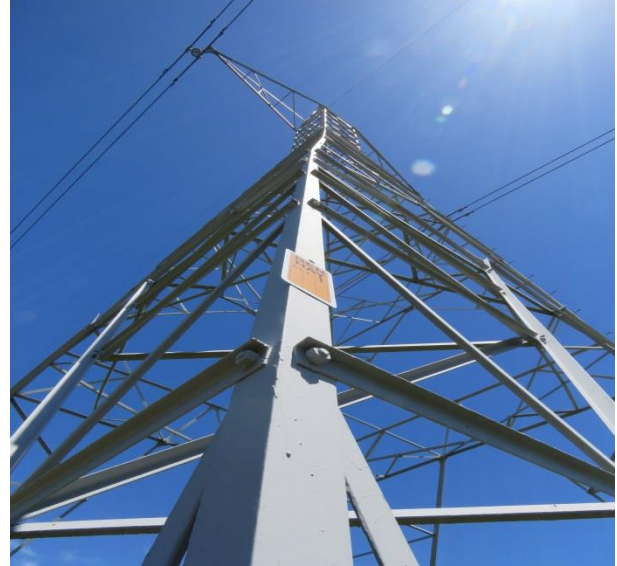
Figure 5: Leg damage of the HVDC Tower.
