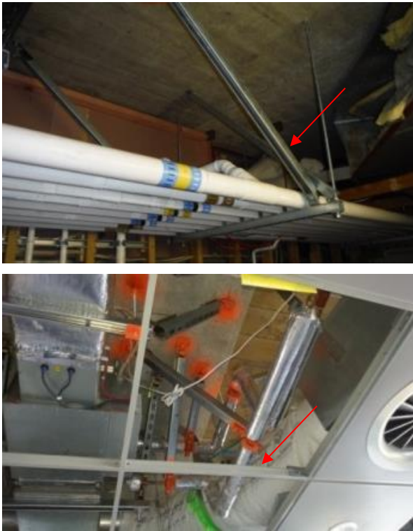
Figure 2: Restraint of new pipework in an existing building on a single trapeze to reduce the number of braces required (top) and new restraint (painted orange) of existing pipework in a modern building (bottom).
