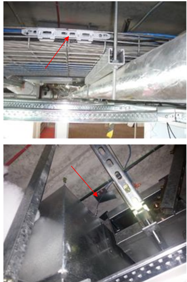
Figure 8: Proprietary seismic clip added to cable tray to strengthen splice (top), wire tether on HVAC kit (bottom).
