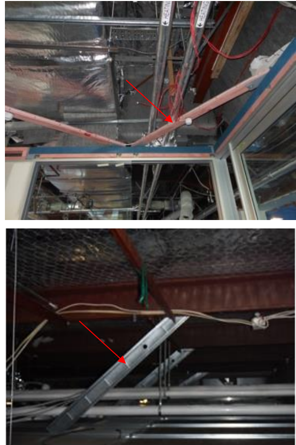
Figure 11: Horizontal bracing above ceiling level (top), restraint of timber partition wall at ceiling level to primary steelwork using tension/compression brace (bottom).
