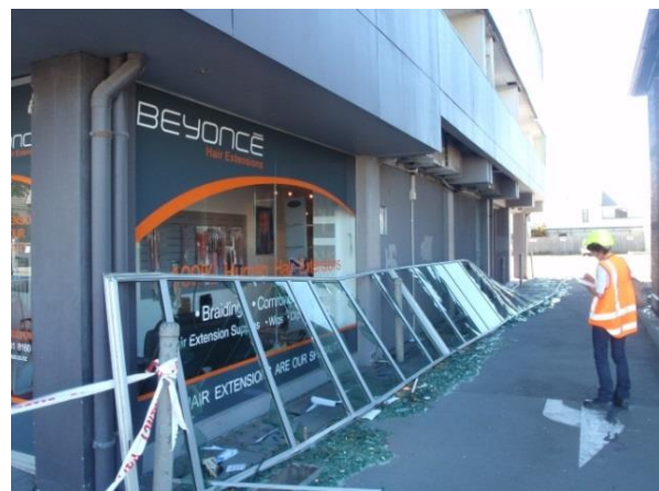
Figure 1: Widespread damage to a ceiling system (top), failure of a lightweight cladding system (bottom).
