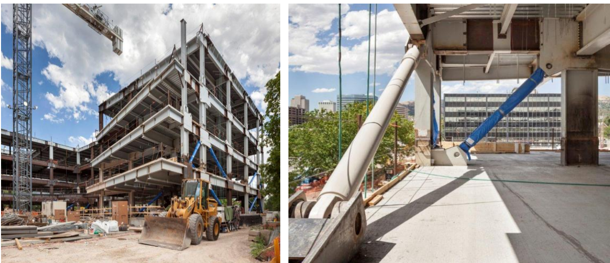
Figure 15: New construction of the Salt Lake City Public Safety Building, a post-disaster performance level steel moment building frame using fluid viscous dampers (Holmes Culley, San Francisco) [5].
