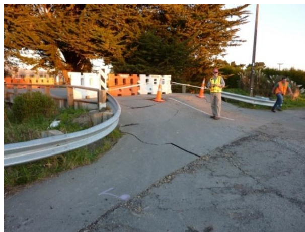
Figure 6: Lateral spreading induced settlement of the western approach.
