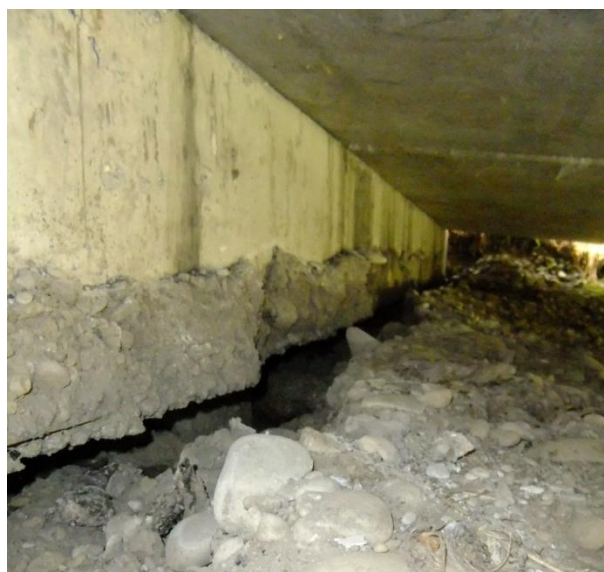
Figure 8: Lateral spreading induced gapping at the pile face of western abutment.
