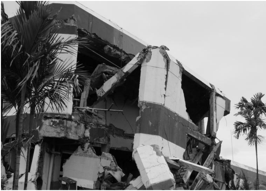
Figure 2. Damage to the main hospital in Padang, Indonesia, after the 30 September 2009 Western Sumatra ( M = 7.6 ) earthquake.
