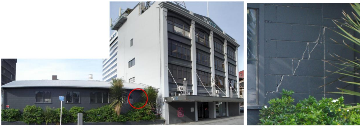
Figure 7: Pounding between 1 storey and 4 storey buildings. Damage to four storey building not attributed to pounding.
