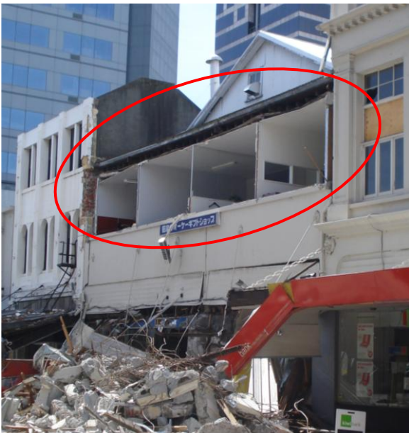
Figure 4: Façade loss attributed to building crushing.
