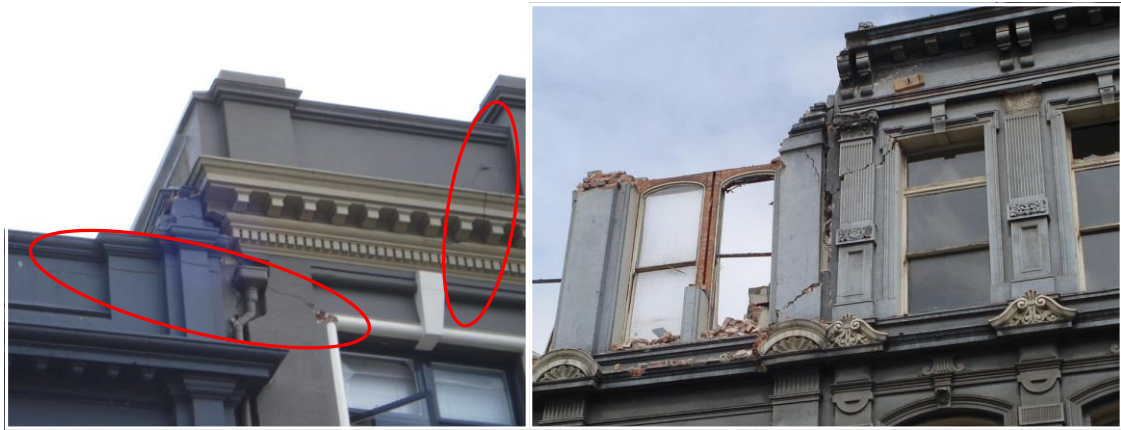
Figure 1: Examples of URM pounding damage. Left: minor damage. Right: major damage partially caused by pounding.
