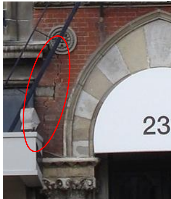
Figure 9: Masonry damage after the Darfield earthquake.
