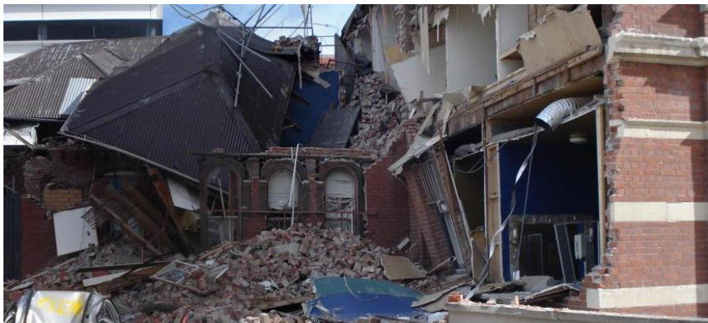
Figure 8: Two storey building collapse involving pounding. Primary cause of collapse is attributed to URM construction.
