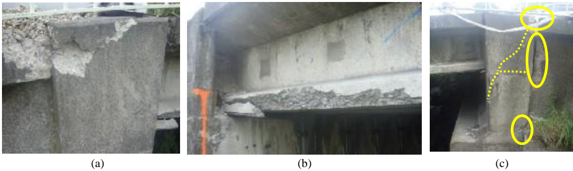
Figure 13: Fitzgerald Avenue Bridge. Pounding damage (a) at the abutment; (b) to the immediate adjacent girder and (c) to the other abutment.
