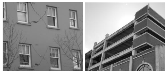
Figure 1: Example of facade damage to masonry infill (left) and precast concrete panels (right).
