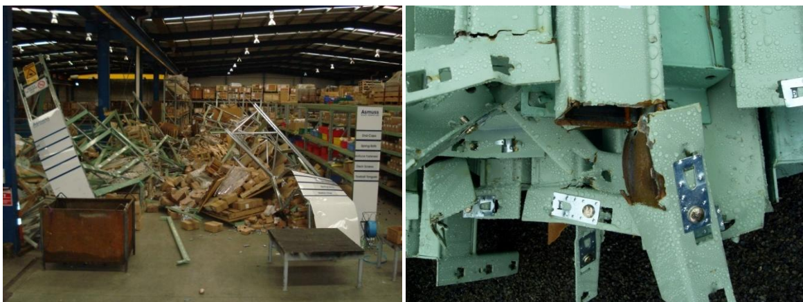
Figure 6: (a) Collapsed racks at metal fabricator and supplier site and (b) fractured connectors from the collapsed racks. Photo credit: N. Crannitch.
