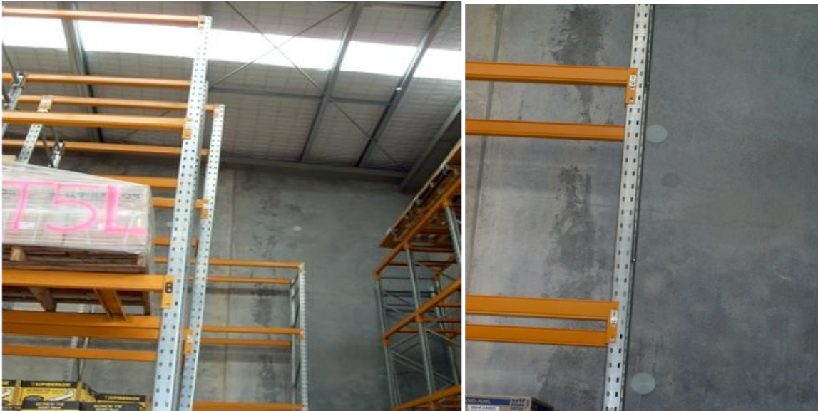
Figure 4: Rack at wood products site with permanent drift. Note relative distances to plugs on wall. Photo credit: D. Mukai.
