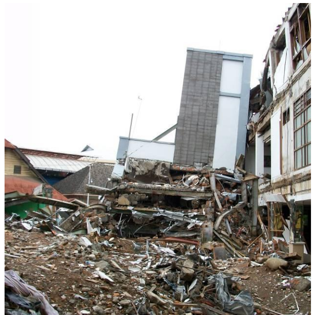
Figure 2: Collapsed 5 level two-way steel MRF addition to hotel.
