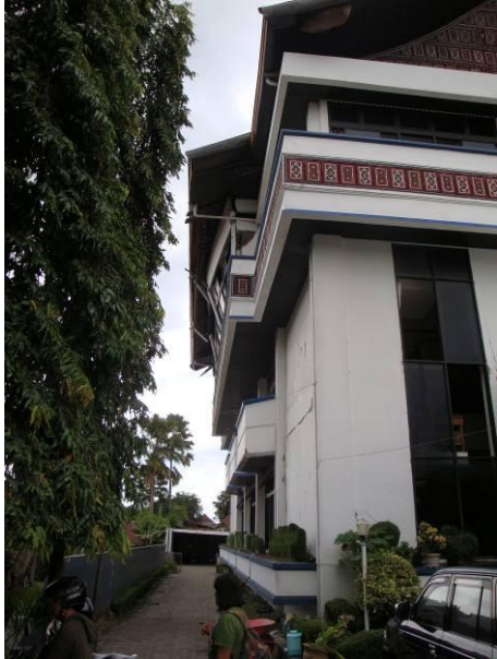
Figure 5: Wall panel detached from roof steelwork above drive way.
