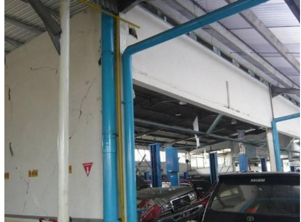
Figure 6: Brick infill panel on steel lintel typical of the type that collapsed under earthquake face loading.
