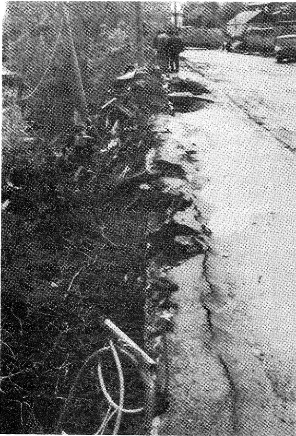
Figure 22 Collapsed wall, Spitak.
