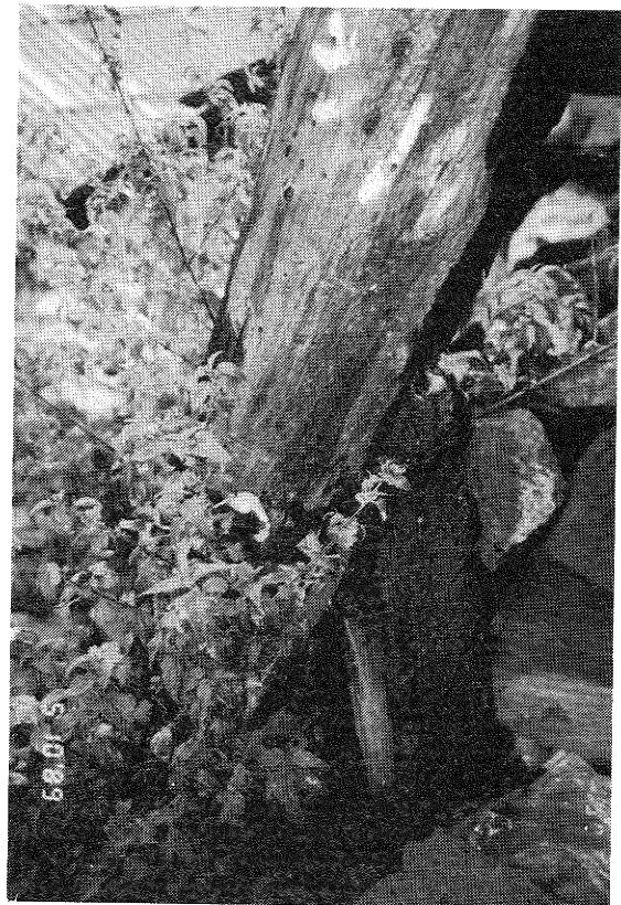
Figure 49 Close up view of power pole fixing failure at Spitak.
