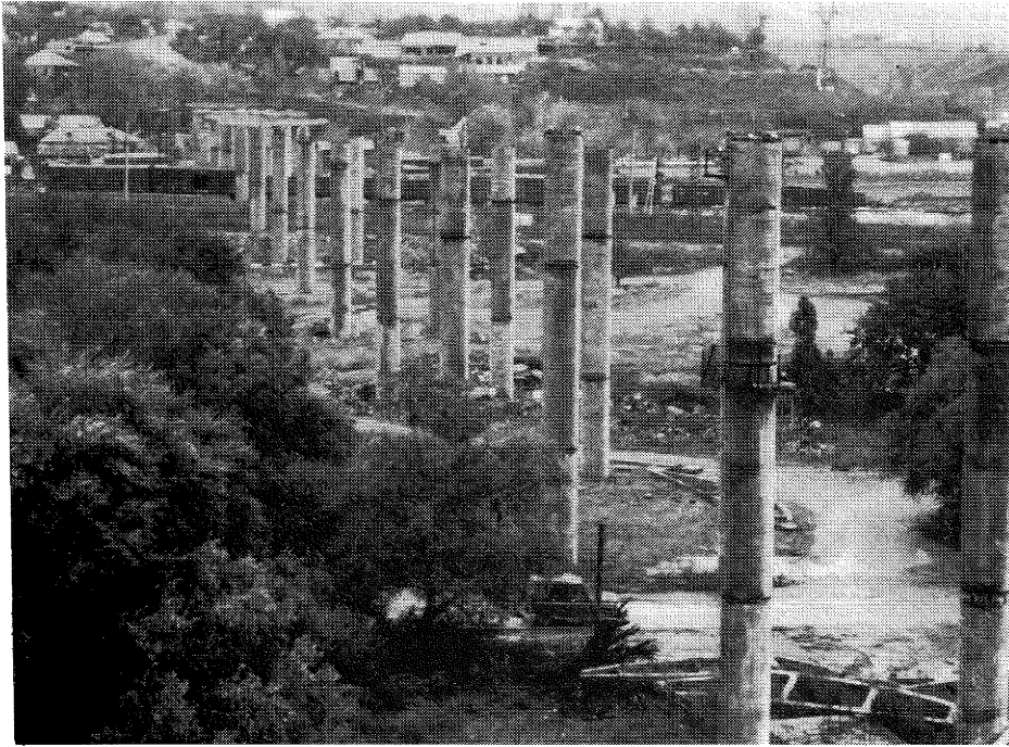
Figure 25 Precast, prestressed concrete highway bridge, under construction at Spitak at time of earthquake.
