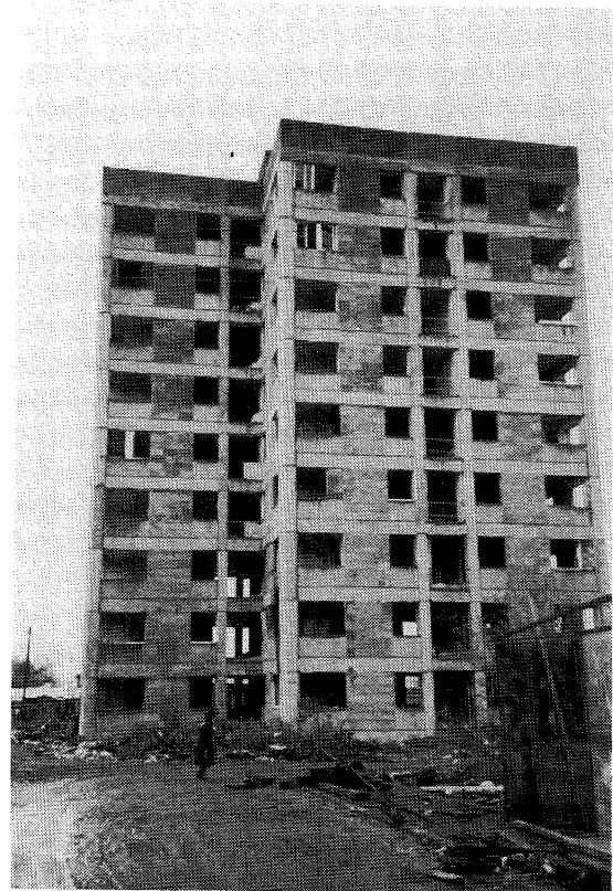
Figure 31 Type 111 building, heavily damaged but still standing, at Leninakan.
