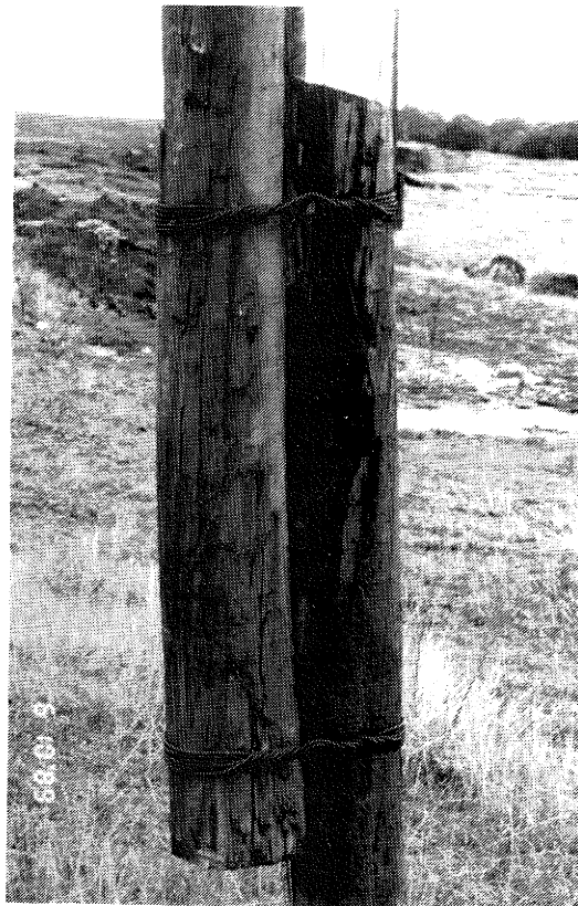
Figure 45 Power pole fixed to timber ground post.
