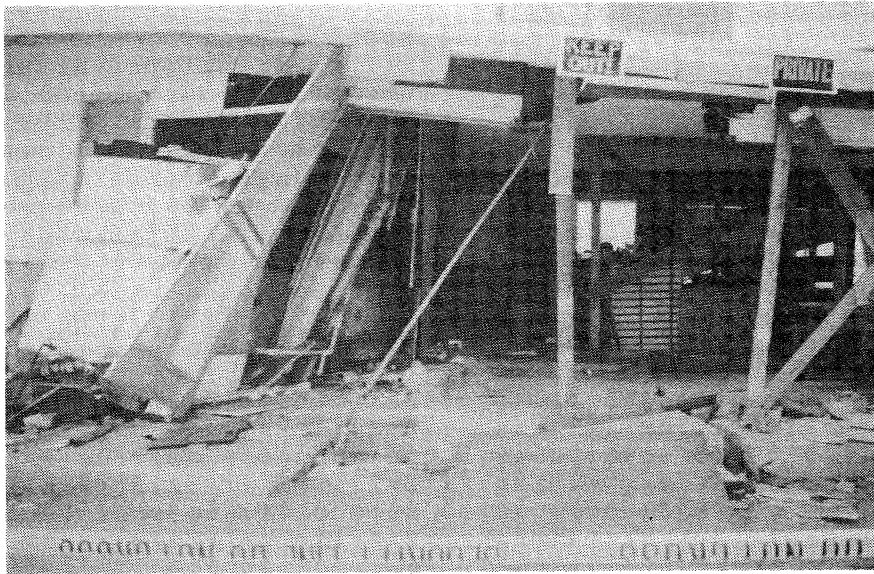
Figure 13. View of the interior of "hilltop" house, showing cracked concrete floor slab, extreme racking of exterior walls (about 1.5 m), and temporary bracing to stop total collapse so that possessions could be removed before demolition.
