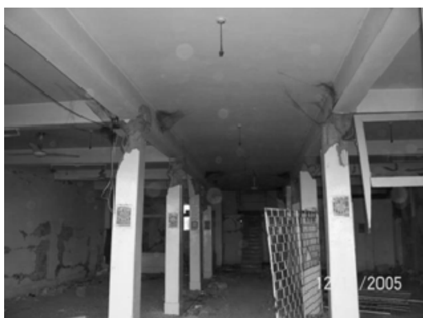
e). Initiation of plastic hinging of columns.
