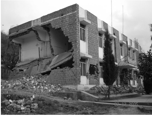
c). A stone masonry building in cement mortar with reinforced concrete floor and roof slab.
