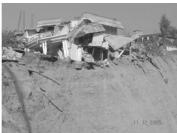
c). Landslide-induced building destruction (Muzaffarabad).
