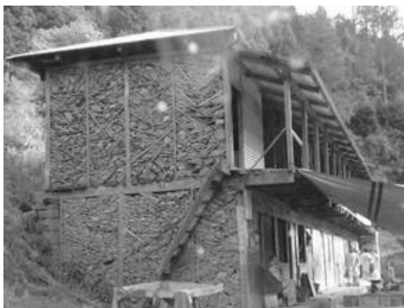
a). Dhajji-dewari that survived the earthquake.
