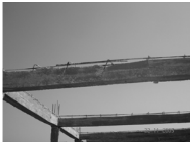
b). A typical reinforced-concrete frame building under construction. (Note: deficient lap length, splice location of column bars; the poorly compacted concrete, and the poorly built frame).
