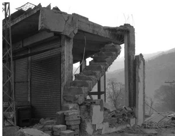
d). Broken waist slab (hanging by reinforcement)
