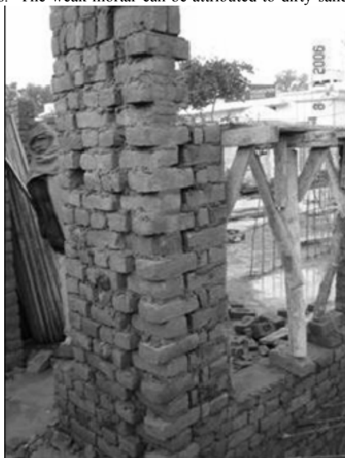
a). Brick masonry house under construction (note the quality of masonry and keys for connection at the wall junction).
