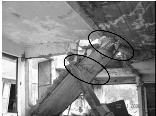
b). Failure due to ending of waist slab and puncture of the floor slab
