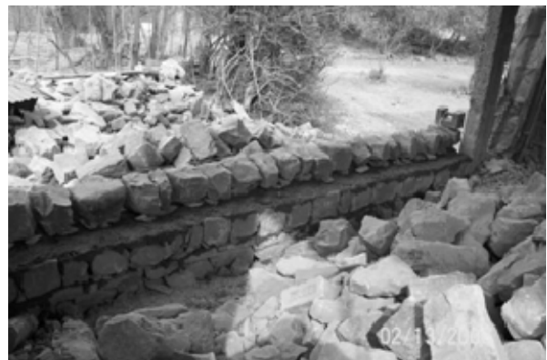
c). Undressed stone wall laid in mud mortar (note that there are no through-stones).
