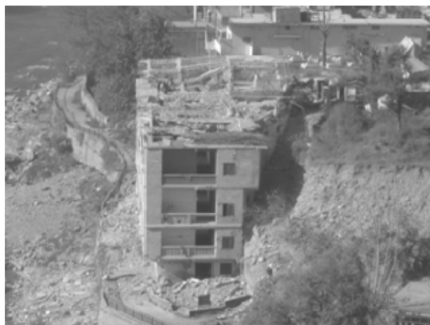
b). Six-storey building abutting hill slope, bottom four storeys abutting hill slope suffered minor to medium damage, whereas top two storeys suffered severe destruction (upper storey under demolition after the earthquake).
