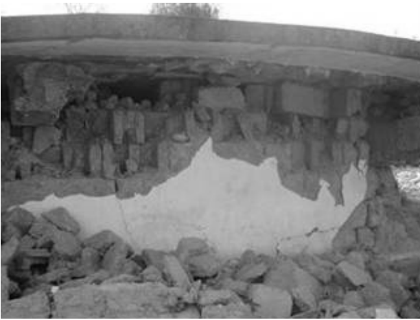
c). Hollow block masonry building (note the crushing of the block shell).
