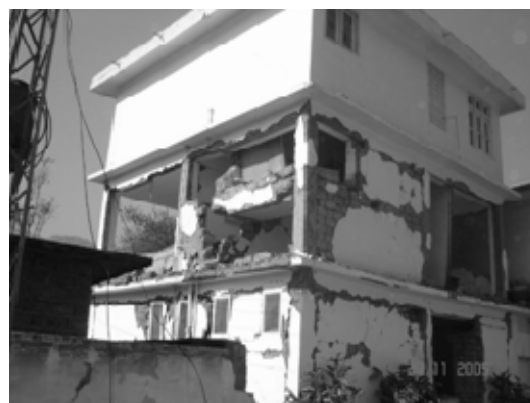
d). Onset of development of soft-storey mechanism.
