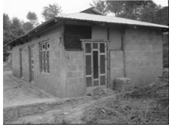
b). A block masonry building with timber frame under construction (after the earthquake).
