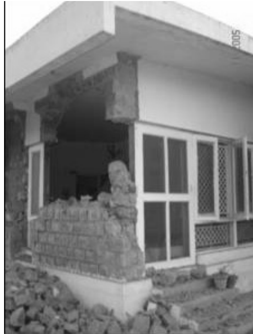
d). Opening in corner-induced damage.
