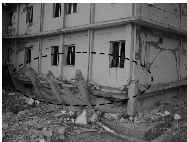
d). Shear failure of first storey columns.
