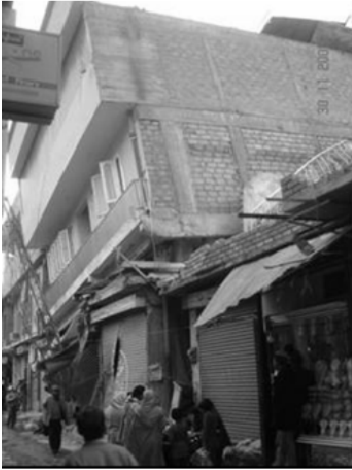
a). Soft-storey failure.
