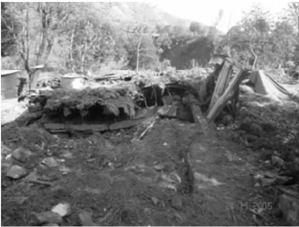
a). Total destruction of Kachcha Makan (note lack of connection between structural components).
