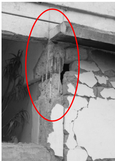
a). A failed column (note that there are not any stirrups for more than 700 mm).
