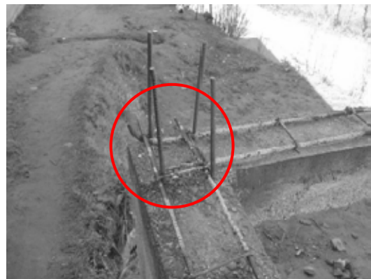
d). Anchorage of beam bars in column (note that there are not any hooks at the ends of bars).
