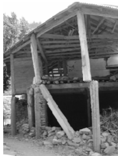
b). A mixed RC frame building in a rural area in NWFP.
