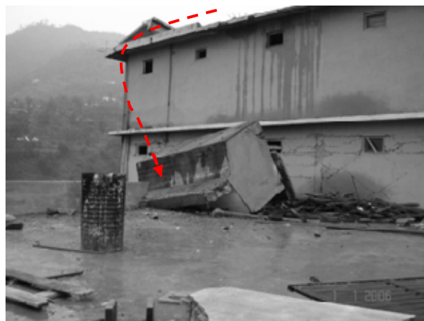
b). A water tank supported on two columns in Muzaffarabad that fell on neighbouring building.
