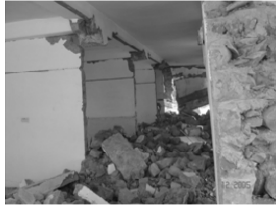
d). Mixing of wall materials (external walls in stone in cement mortar, external walls in concrete blocks).
