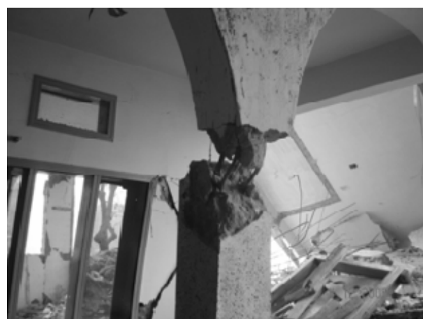
f). Failure of column due to sudden change of stiffness.
