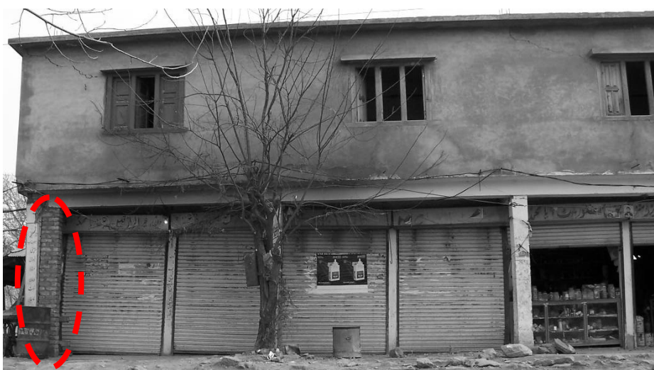
Figure 12. Masonry columns instead of reinforced concrete column.
