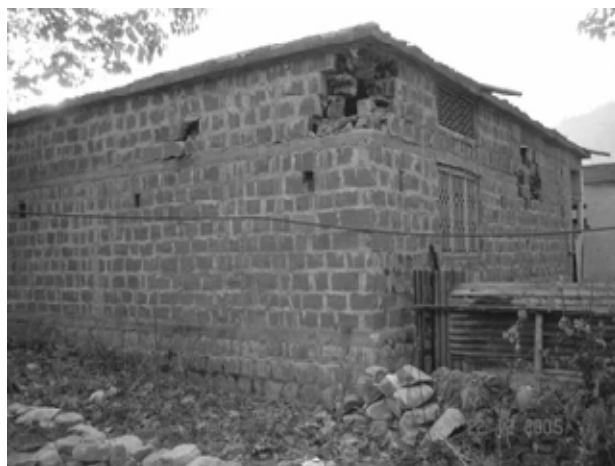
b). Falling of stones at the corners and where the band level is split.
