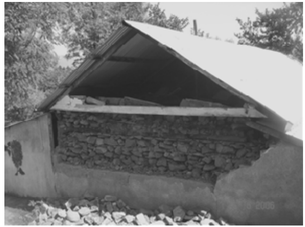
b). Delamination of a stone wall, and out-of-plane collapse of the gable wall.
