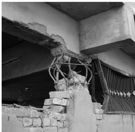
b). Short-column effect due to partial height masonry – surprising that the bars have not fractured.
