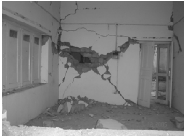
d). Sliding failure of brick-masonry wall.
