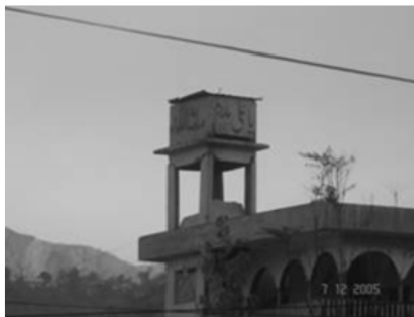
a). An elevated water tank in Muzaffarabad (note development of cracks at the top of columns).
