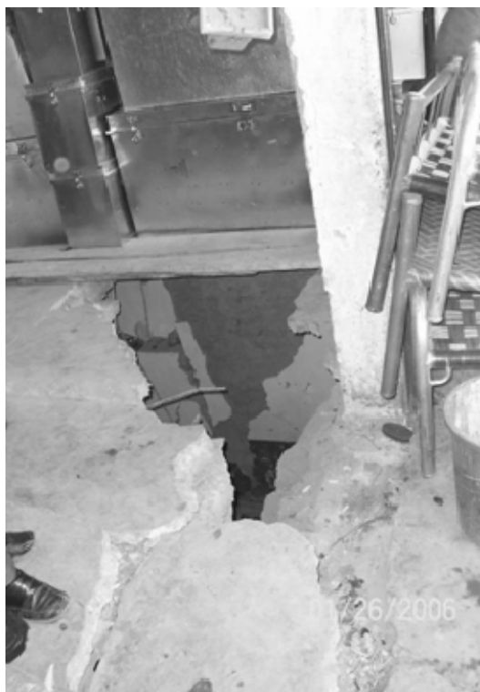
c). RC slab of second floor with almost no reinforcement.
