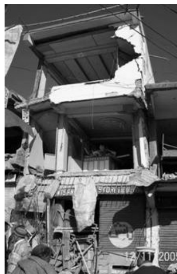
f). Out-of-plane failure of masonry in RC frame building.
