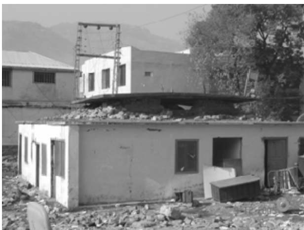
Figure 4. Destruction of second storey of a stone masonry building without lateral displacement.
