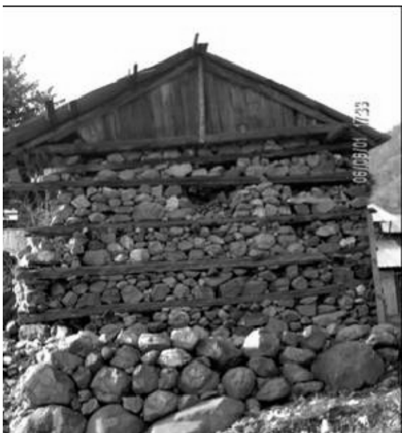
a). Batar in round rubble masonry survived earthquake with localised damage.
