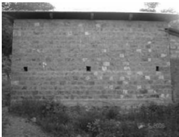
a). Excellent seismic performance presumably due to a reinforced concrete band at eaves level in Muzaffarabad.
