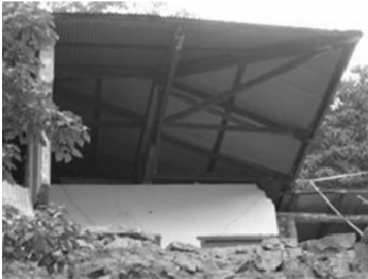
a). Hipped roof standing even after collapse of supports.
