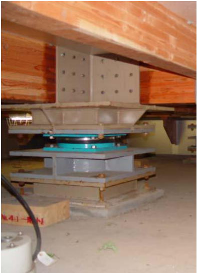
Figure 6: Base isolator under timber building (Sakamoto et al. 1990)
