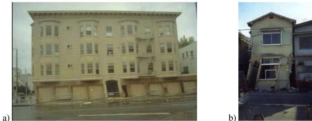
Figure 1: Soft first story in a) Loma Prieta (ATC 2009) and b) Kobe earthquake (Ghosh 1995)
