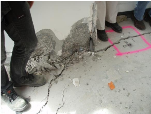
Figure 5.1: Precast floor damage at Clarendon Tower
