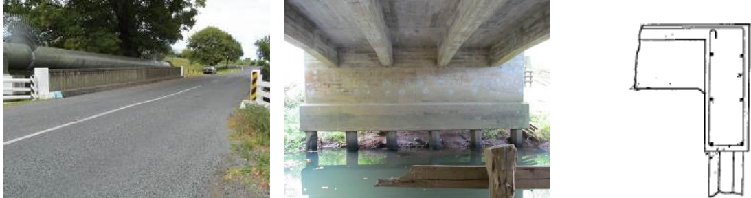
(a) Deck with concrete barriers (b) Wall pier with scour exposed (c) Abutment detail piles.
