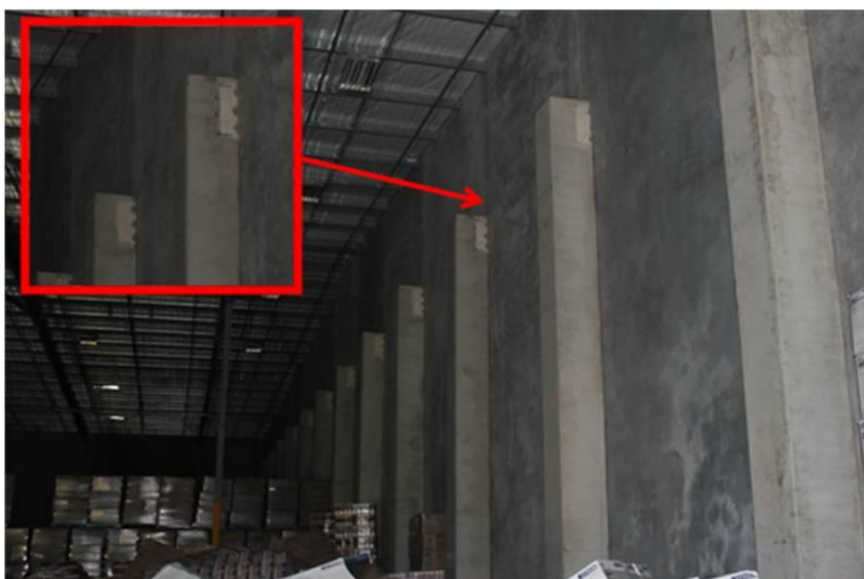
Figure 4. Example of ductile cast-in anchors as part of the main lateral load-resisting system demonstrating good performance under seismic actions. Inset: spalled vermiculite fire-rating material showing evidence of movement of the connection under seismic actions
