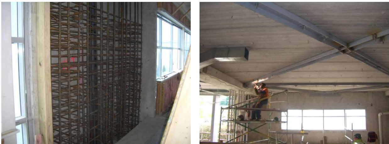
Figure 2. Repair and upgrade of Statistics New Zealand: a) New in situ reinforced concrete shear walls; b) Diaphragm strengthening using steel bracing to underside of floors
