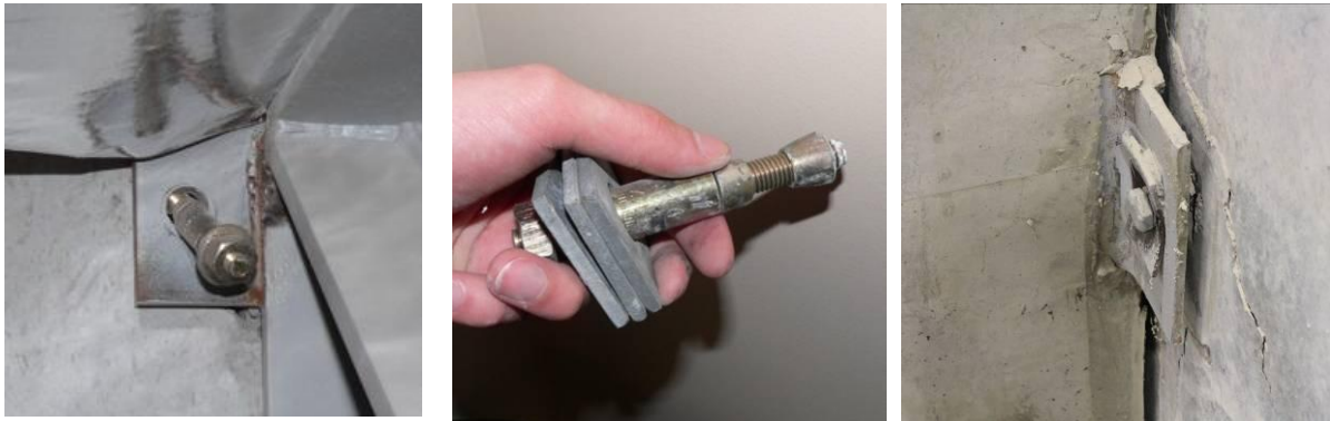
Figure 5. Examples of performance of bolted panel connections: a, b) Pullout of expansion anchor; c) Ductile cast-in anchor showing surface panel spalling
