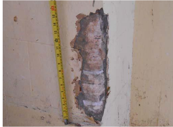
Rectangular-shaped stone and debris embedded in mortar
