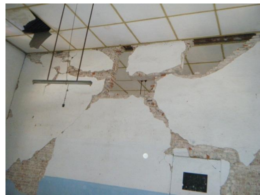
Figure 5. Shear cracking in infill wall material.
