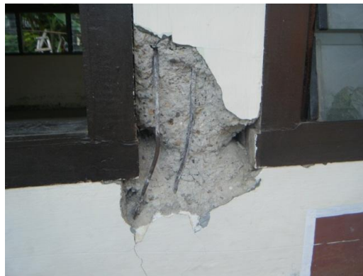
Figure 2. Poor reinforcement detailing with a lack of transverse reinforcement and insufficient longitudinal reinforcement.
