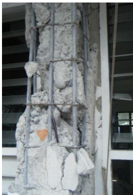
Figure 1. Poor quality concrete material is vulnerable to crushing and shearing.
