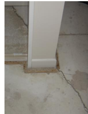
Figure 5. Cracking in floor slab.
