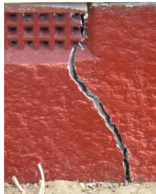
Figure 4. Typical crack in concrete perimeter foundation.
