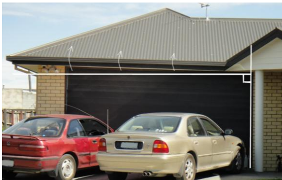
Figure 6. Differential tilting of garage of slab-on-grade house.
