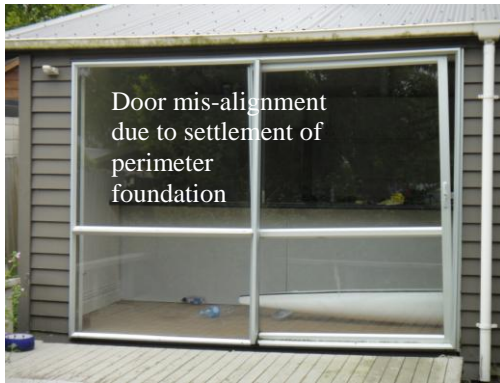
Figure 3. Damage caused by racking in a house, showing door mis-alignment.
