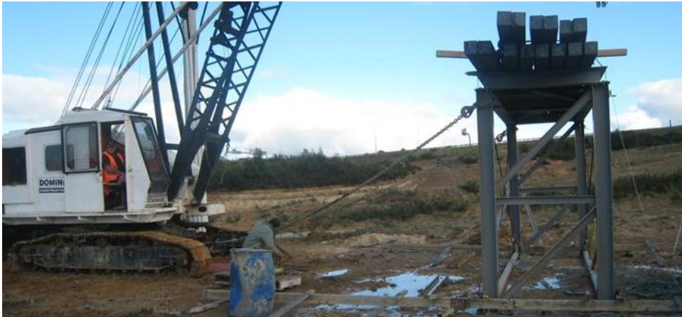
Figure 1 Shallow foundation set-up for snap back testing. Simple structure loaded with kentledge and supported on shallow foundations at the right. Chains attached to a hydraulic ram with a quick release shackle connected to the crane to provide reaction.
