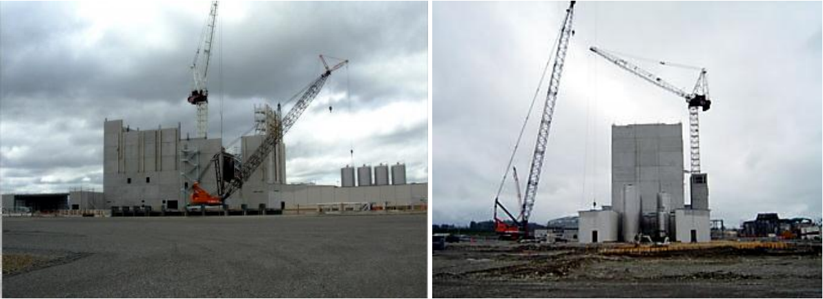
Figure 3: Fonterra Darfield Dryer Plant during construction (courtesy DLA Architects and Ebert Construction)
