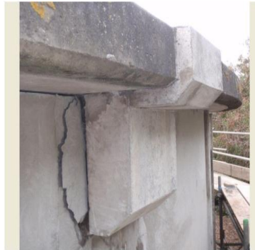
Figure 5 - Upper Balmoral wall damage
