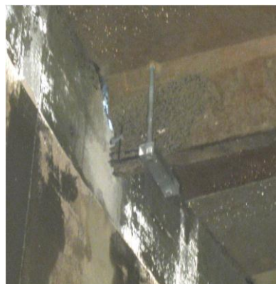
Figure 2 - McCormacks roof / wall impact damage
