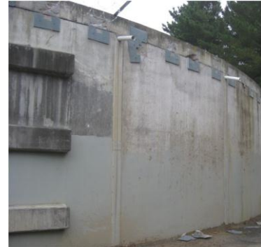
Figure 6 - Worsleys Rd reservoir No.1 epoxy bonded shear plates
