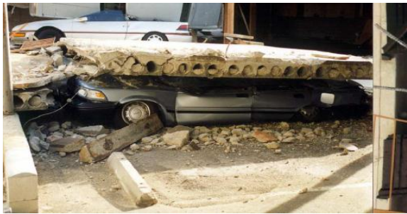
(b) Collapse of hollow-core flooring unit following 1994 Northridge earthquake (Norton, King et al. 1994).
