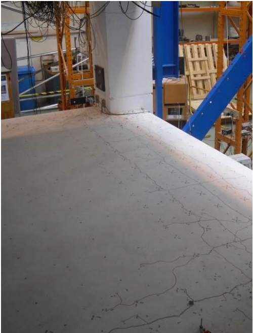
(c) Timber infill cracks, all less than 0.45mm.
