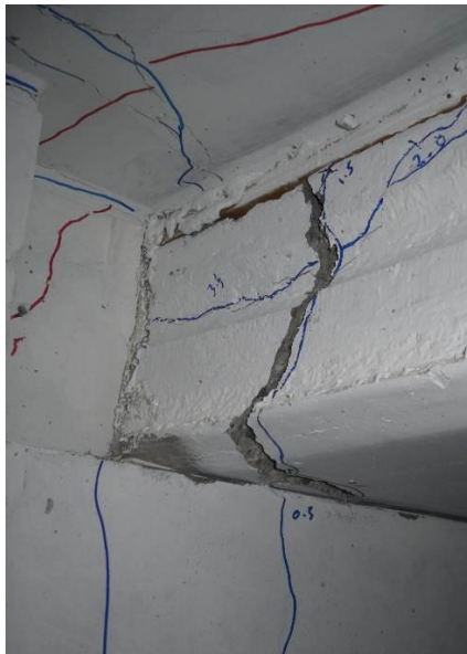
(a) Cracked end.
