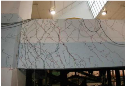
(a) Example of fully formed plastic hinge zone (Matthews 2004).
