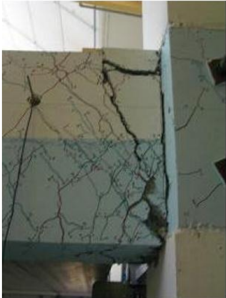
(b) Monolithic reinforced concrete plastic hinge damage (MacPherson 2005).
