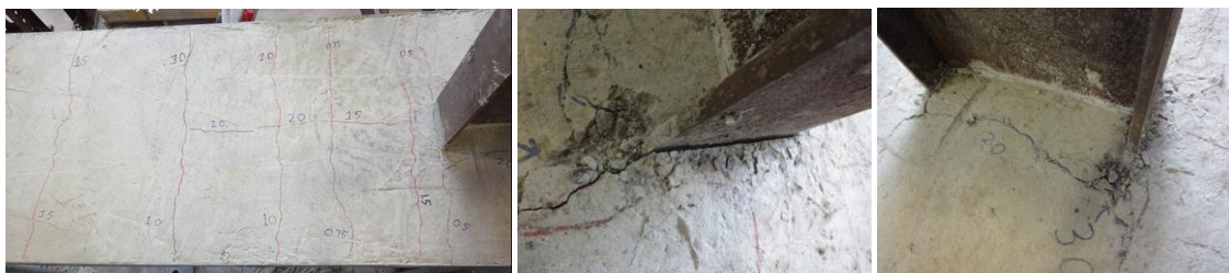
Figure 5: Left to right: Pattern of slab cracking, column face at 3% drift and cracking at column base
