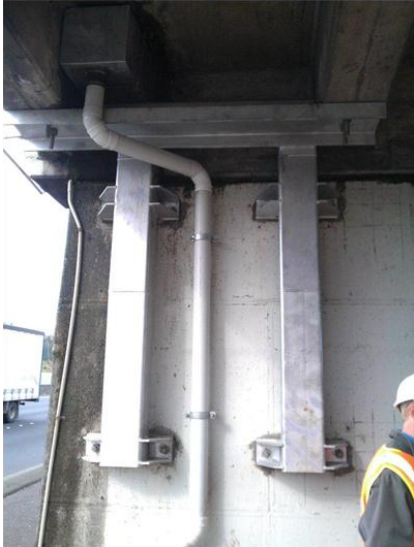
Figure 17: Shear keys at the Off-ramp abutment – working around existing services is always a joy
