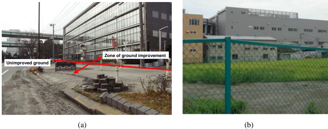
Figure 5: (a) Excellent performance of SCP-improved ground in Tatsumi; and (b) an undamaged building resting on improved ground in Shin-kiba while adjacent to it, sand boils were everywhere.
