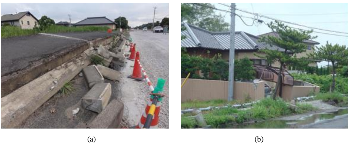
Figure 6: (a) A portion of the road in Kamisu City which settled due to liquefaction; and (b) damaged house as a result of liquefaction in Itako City.
