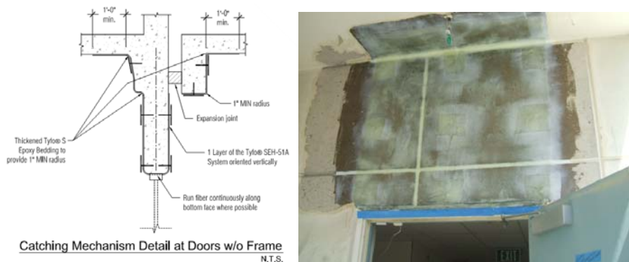
Figure 6. Spandrel walls over doorways were wrapped with the Tyfo ® SEH Composite System to act as a life safety catch mechanism during seismic events.
