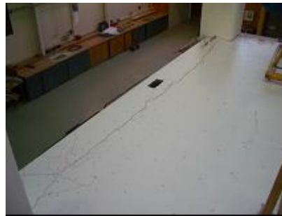
(b) Continuity crack after Phase I.
