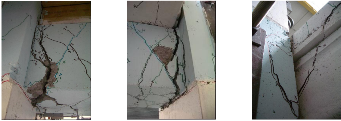
(a) Damage to the south end of the west transverse beam at +3%. (b) Damage to the north end of the west transverse beam at +3%. (c) Hollow-core web cracking and damage at the north east corner after Phase II testing.
