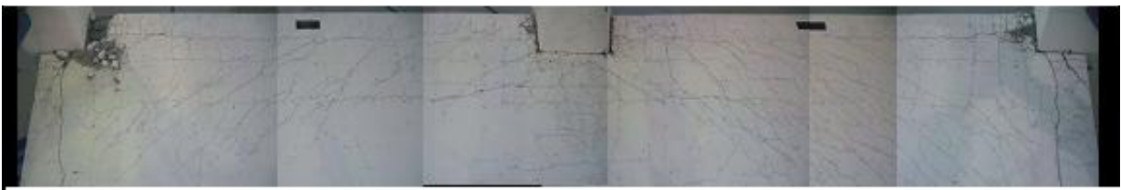
Figure 6. Floor damage after the completion of testing.
