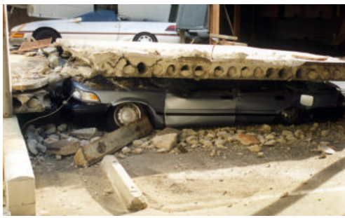
(a) Complete collapse of a floor slab
