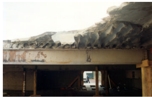
(b) Partial collapse of a floor slab.
