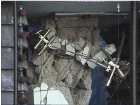
Figure 5b. Top of center column, Specimen 2 at end of test
