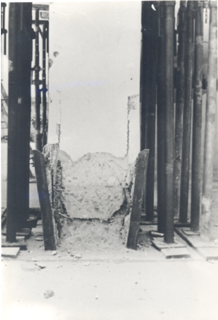
Figure 1(b): San Bosco, damage at the base of a first-storey corner column.
