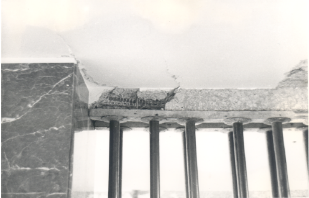
Figure 2(b): Residencia Union, damaged end of a first storey beam.
