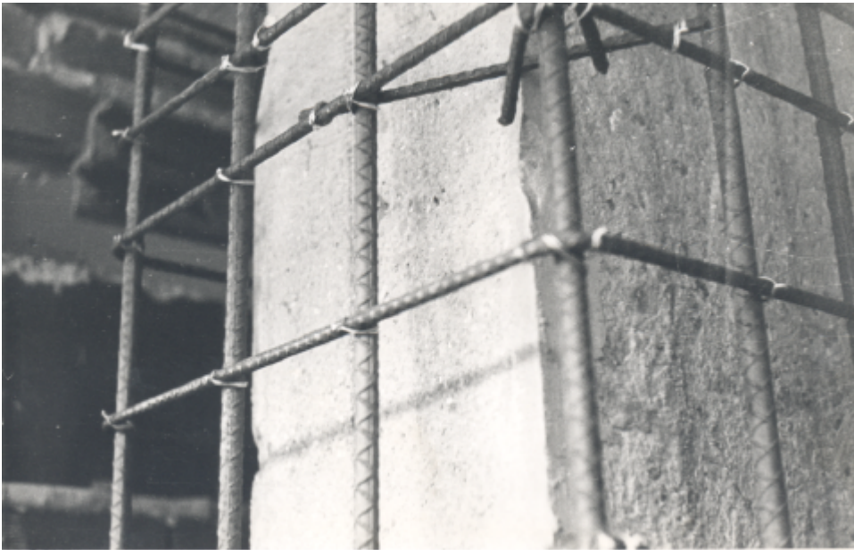
Figure 1(c) : San Bosco, reinforcing steel for the upgrade of a first storey column.
