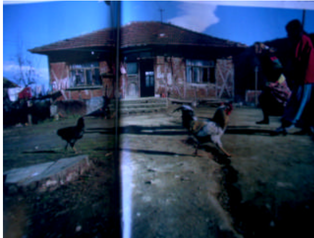
Figure 1: A traditional building with minor damage. Note ground failure in foreground of house (source: National geographic, July 2000).
