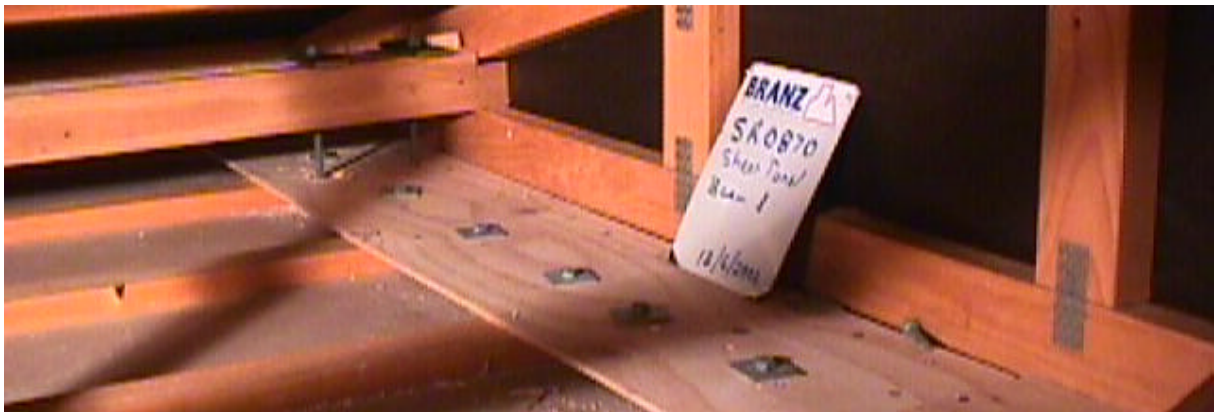
(c) Plywood strip in roof space to connect timber loading beams to wall top plate
