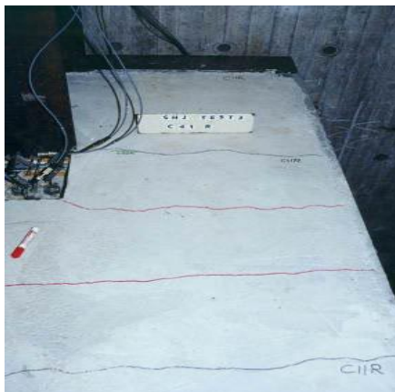
Figure 9 SHJ test 3: Condition of concrete slab at design
